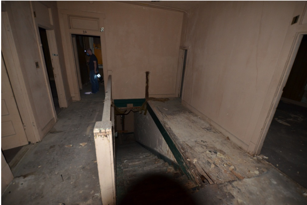
Figure 3: Second floor, central hall, looking west. Photographer: Kris Calvert, CMA Architecture, November 2009.
