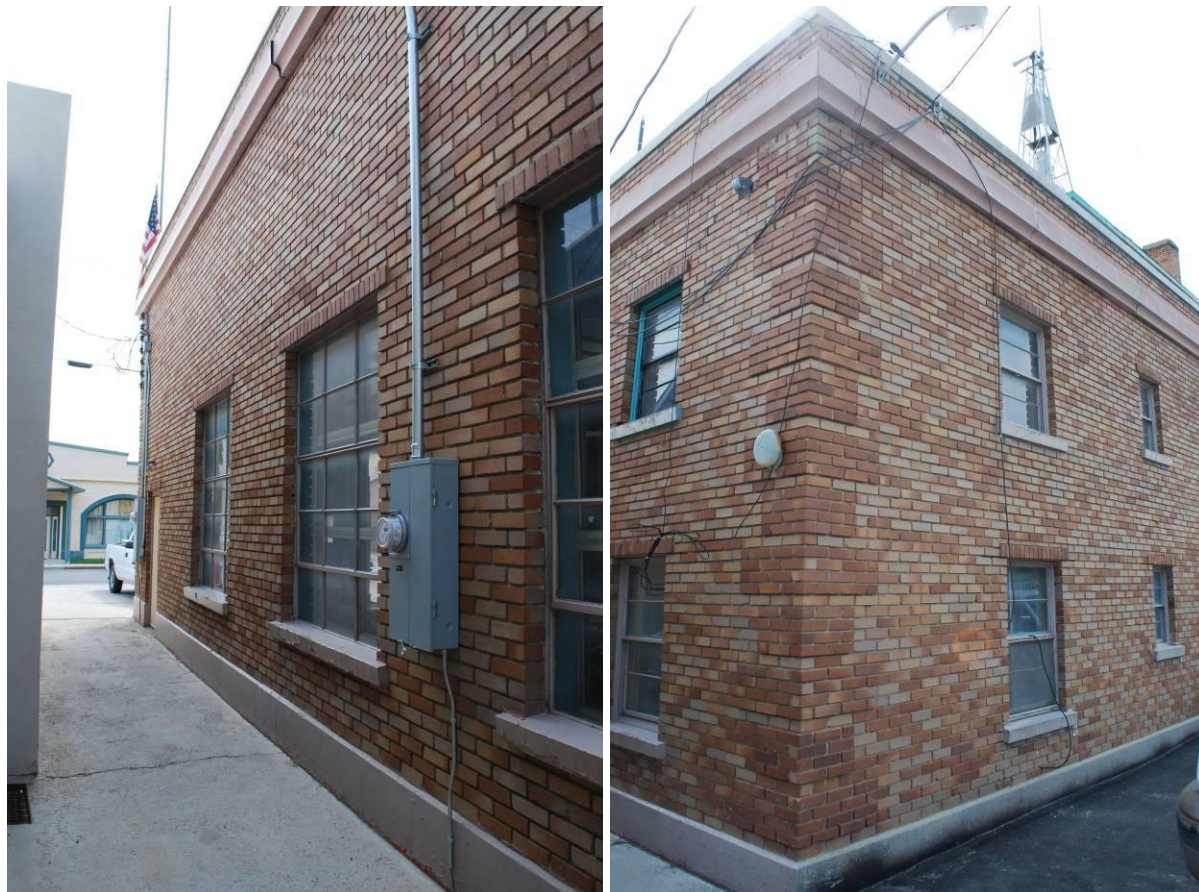
Photograph 2 and 3 – Northwest corner, looking southeast, showing north (left) and rear (right) elevations (NVSHPO, 2015).
