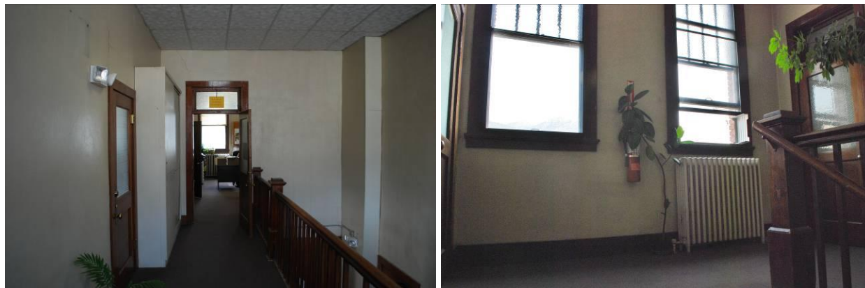
Photograph 8 and 9: Looking north down 2 nd floor hallway (left); Looking up stairwell to south windows (right) (NVSHPO 2015).
