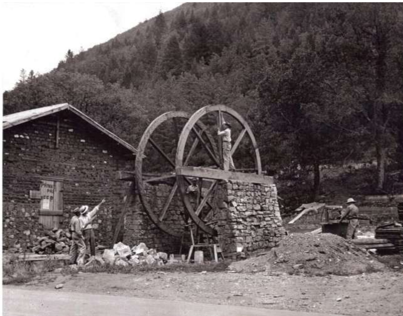
Figure 14 Vintage Photo 14 of 16, circa 1950, Rebuilding water wheel, camera facing southeast Carmon Phillips Collection
