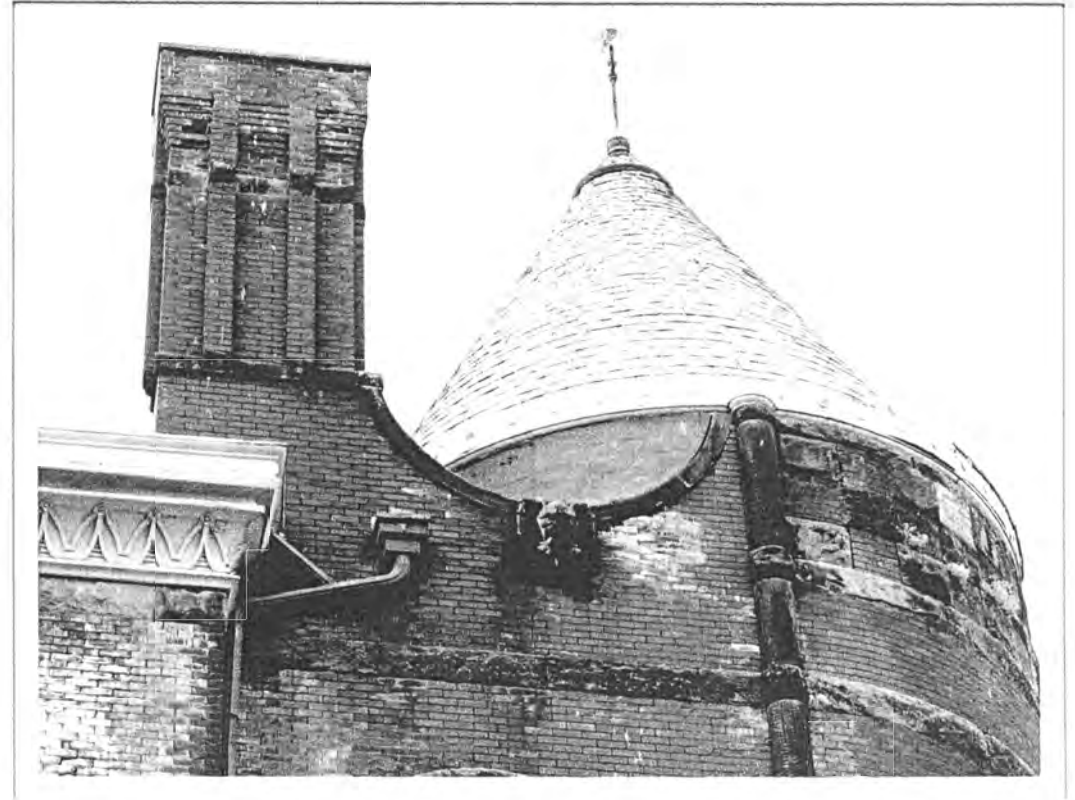
Photo 6 (below) The Cox Building, MS-M-III, Mason County, Ky. Detail Tin Cornice, Slate Tower, Brick Chimney, Stone "Green Man" & Checkered Pattern. Looking S Orloff Miller, 2007, author's collection.
