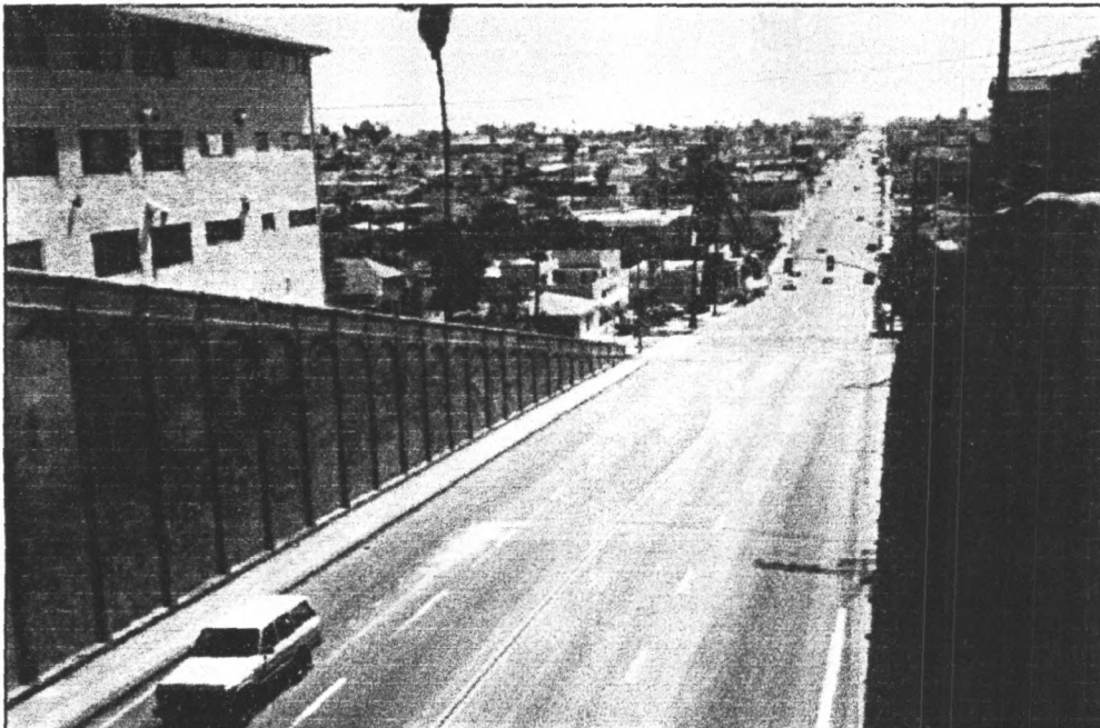
Photograph #5 Georgia Street Bridge/University Avenue Grade Separation Cut Retaining Walls San Diego County, CA Photograph Taken by Alex D. Bevil May 1998 Original Negative in Possession of Photographer View of Eastern Approach to Bridge, Looking East from the Bridge's Deck toward the Intersection of University Avenue and Florida Street
