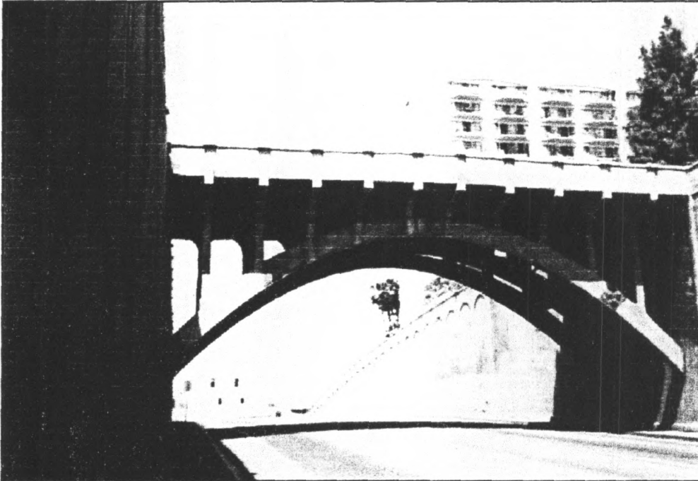
Photograph #6 Georgia Street Bridge/University Avenue Grade Separation Cut Retaining Walls San Diego County, CA Photograph Taken by Alex D. Bevil May 1998 Original Negative in Possession of Photographer Close-up View of Eastern Approach to Bridge, Looking West toward the Intersection of University Avenue and Park Boulevard
