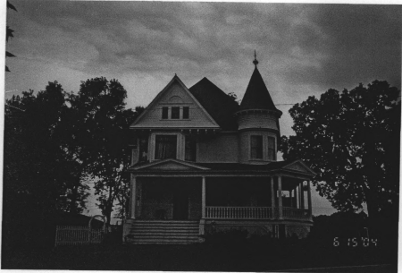
Figure 1: Corner of South 14 th Street & 2 nd Avenue South (intact other than chimney is missing; house needs significant maintenance -- paint is peeling and roof has loose shingles, rating of 8).
