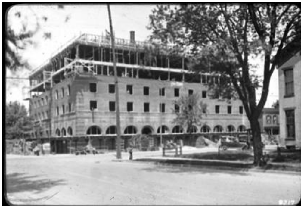
Figure 14. Ca. 1922 photograph of Hotel Manchester under construction in Middletown, Ohio, looking northwest
