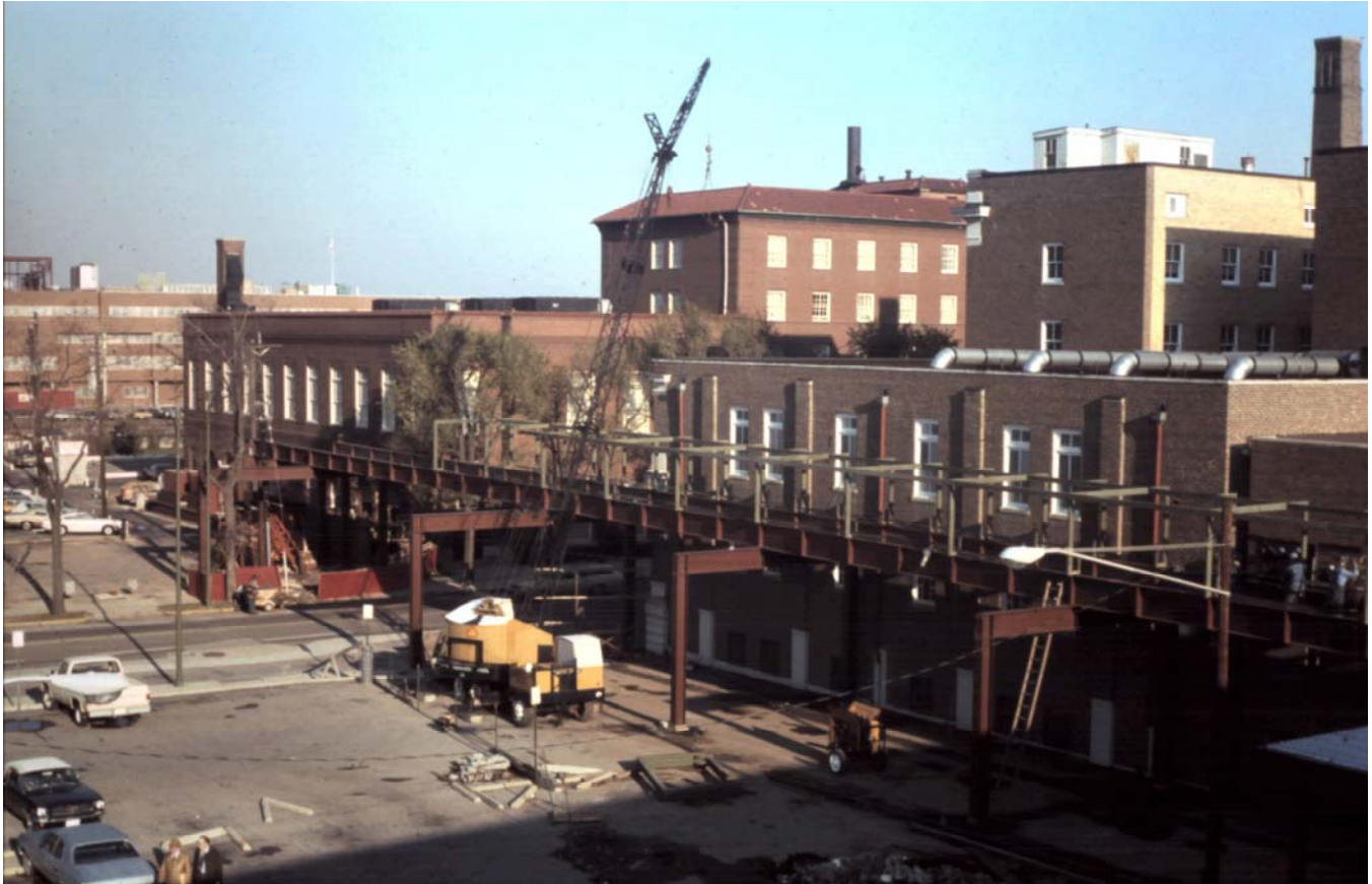
Figure 18. Ca. 1975 photograph showing construction of walkway that formerly connected the Hotel Manchester to a parking garage and the YMCA building in Middletown, Ohio, looking northeast Source: George C. Crout Collection, MidPointe Library System, Middletown, Ohio
