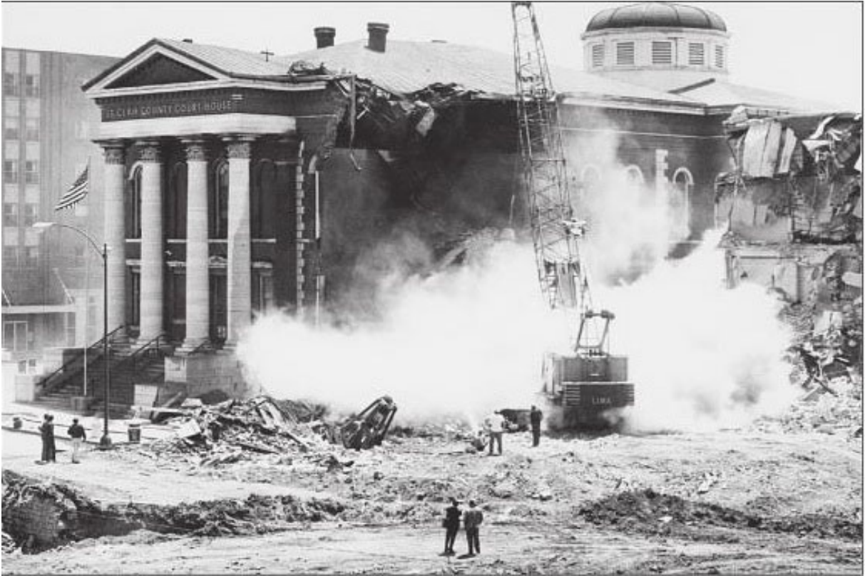
Figure 3: Photograph of the St. Clair County Courthouse under demolition, 1972. Source: Belleville Historical Society.
