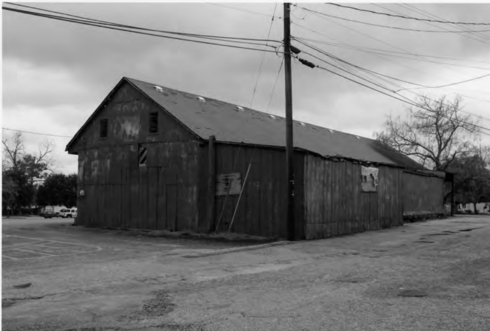
36. Manning Commercial Historic District 15 East Boyce Street, Manning Clarendon County, South Carolina
