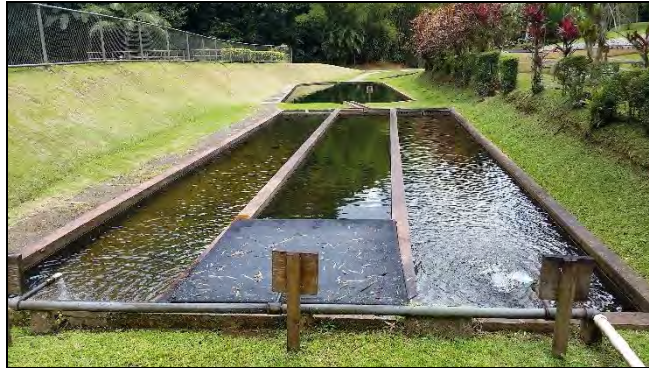
Picture 17. View of the retention tank’s (T26-T28) three pools. Photo taken from the Gazebo area looking east.
