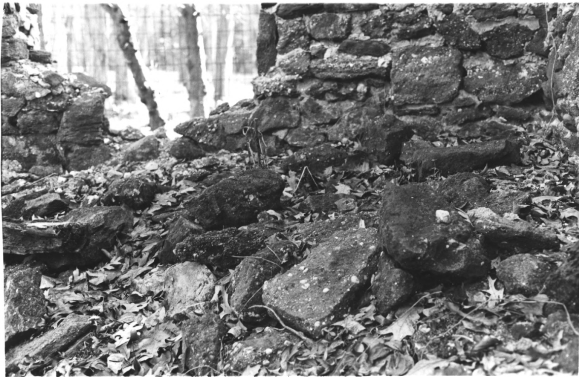
10. Pot House Site/Estellville Glassworks H.D., Estell Manor City, Atlantic County, New Jersey
