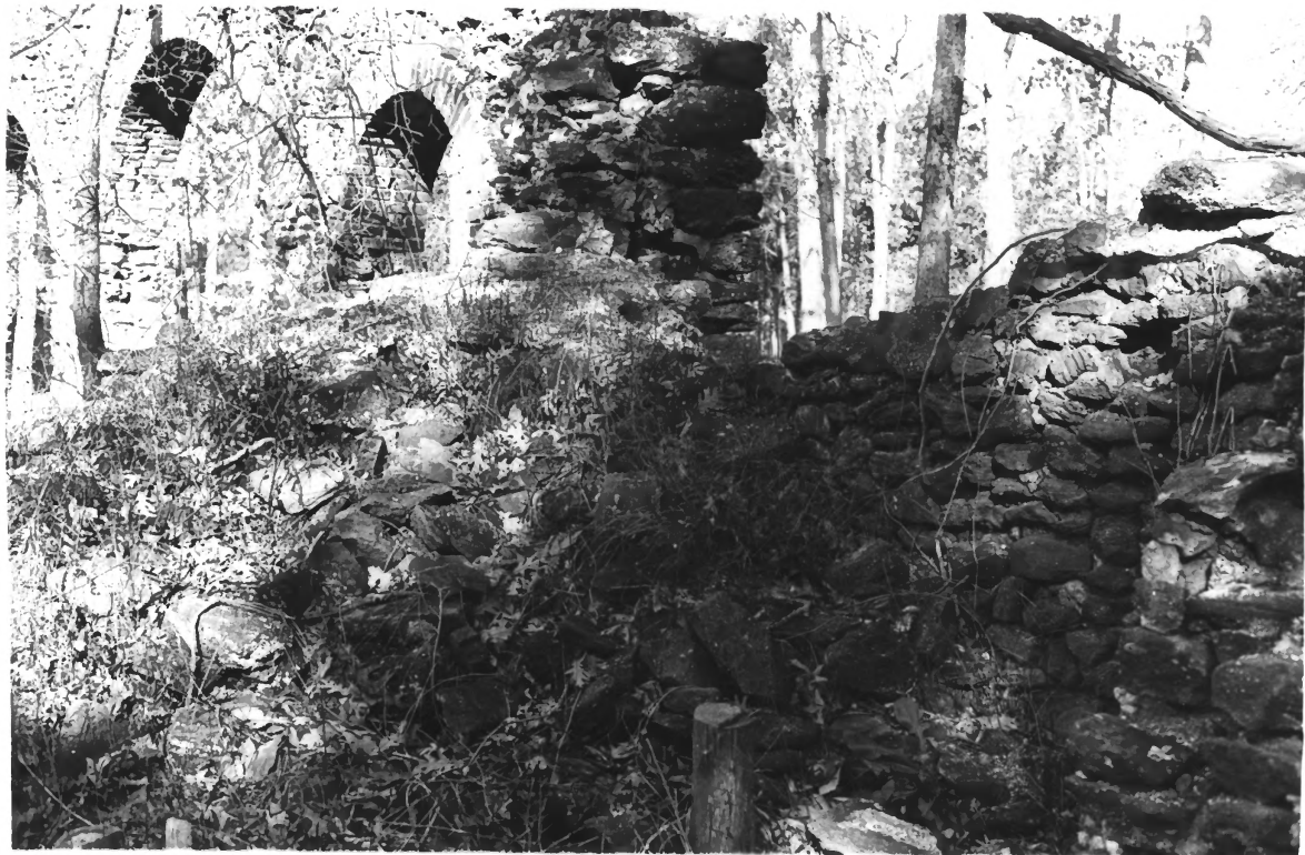
5. Melting Furnace Site / Estellville Glassworks H.D., Estell Manor City, Atlantic County, New Jersey
