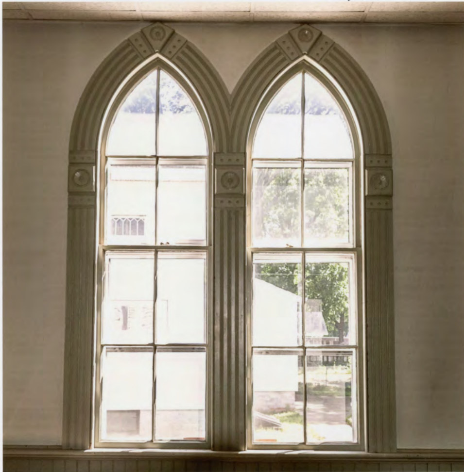
photo 20. Plainville Congregational Church, Plainville, Hartford County, Connecticut. Music room addition interior, view south showing lancet windows and moldings. October 29, 2011, Tod Bryant
