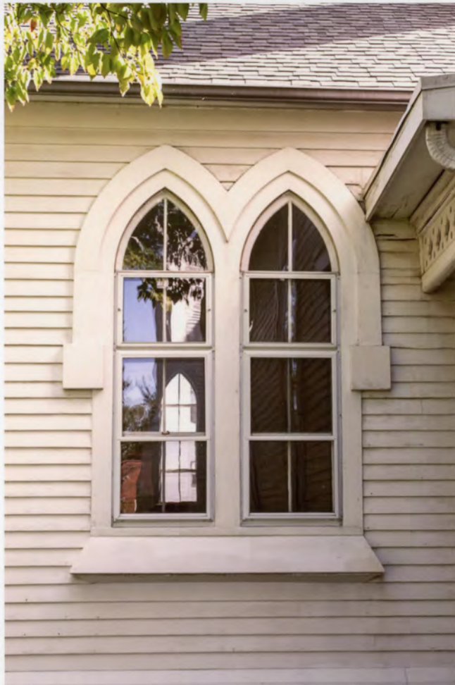
Photo 7. Plainville Congregational Church, Plainville, Hartford County, Connecticut, view south, Music Room addition, north elevation, showing paired lancet windows. August 29, 2011, Tod Bryant.
