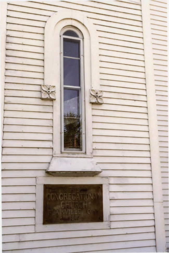
Photo 6. Plainville Congregational Church, Plainville, Hartford County, Connecticut, view south, tower, north elevation, showing round headed window and fluted bosses. August 29, 2011, Tod Bryant.
