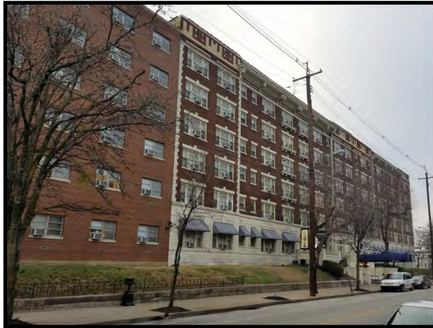
Figure 10. Closer view of 1914 and 1925 portions of the building's primary façade, looking northwest. The 1958 addition is in the foreground. (Photo 0007).
