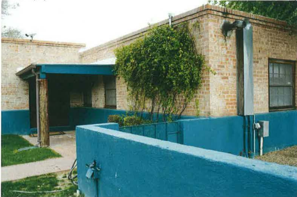
Photograph 7. Detail of wall and gate around courtyard, southwest corner (A.T. Willett 2017) (AZPimaCounty_WoodrowResidence_007).
