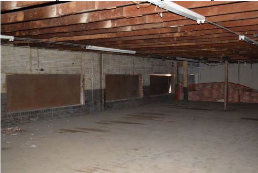
Photo 16: 2 nd floor tire storage area, over service area. Showing the north facing windows. Camera facing northeast.
