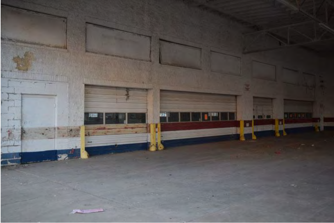
Photo 9: Service station entrance and garage doors (located beneath canopy). Camera facing southwest.
