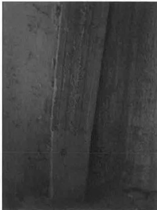
Photo 6: Built-up post showing first-level deflection
