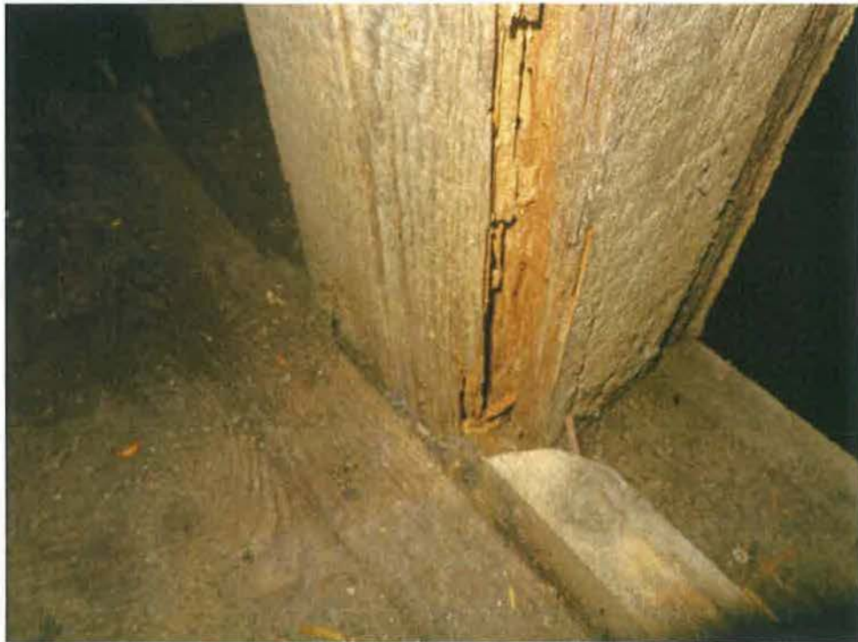
Photo 10: Dry rot at bottom of roof post.
