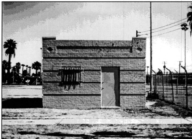
This enhanced photograph shows how the building might have looked without the infilling of the lower three recessed courses of brick.
