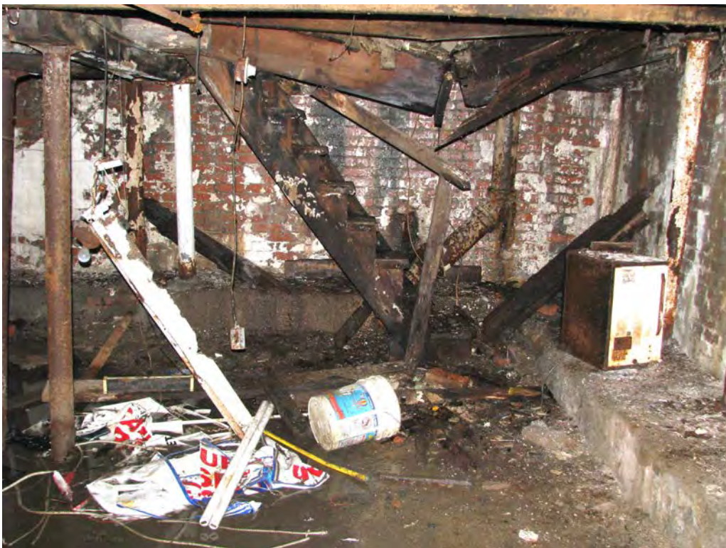
Photo 30. Basement, looking north at collapsed stair to kitchen above (P+A, 2018).
