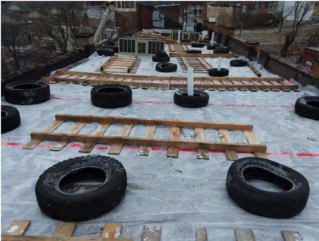
Photo 31. Roof, looking north, showing temporary roofing with stair penthouse in background (Rob Pfaffmann, Pfaffmann + Associates, P+A, January 2018).
