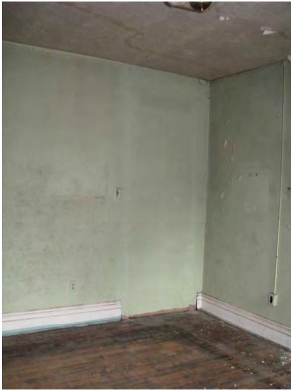
Photo 22. Second floor, rear apartment, looking northwest, showing one of the doors that had been concealed (P+A, 2018).
