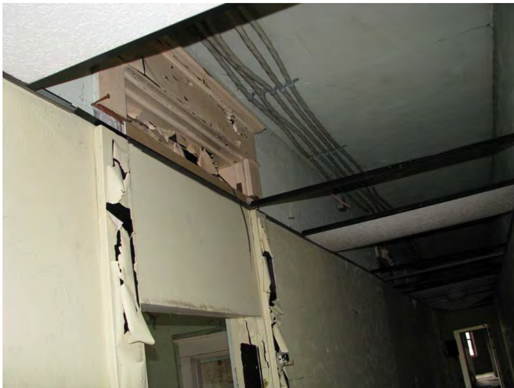
Photo 21. Second floor, looking southeast in the corridor, showing one of the transoms that had been concealed (P+A, 2018).
