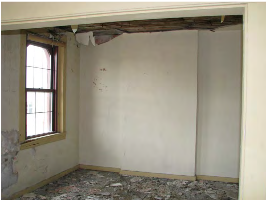
Photo 28. Third floor, bedroom in the front apartment, looking west, showing the projecting chimney breast that once contained a fireplace mantel (P+A, 2018).
