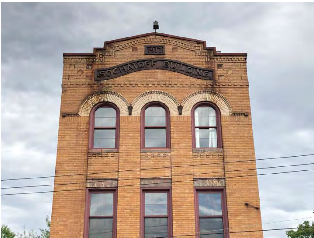
Photo 6. Upper stories of the front facade, looking north, showing the ornate cornice and carved stone date and name banners (T&P, 2019).
