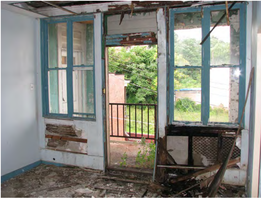
Photo 27. Third floor, living room of the front apartment, looking east, showing access to the shared recessed porch and former fire escape egress (P+A, 2018).
