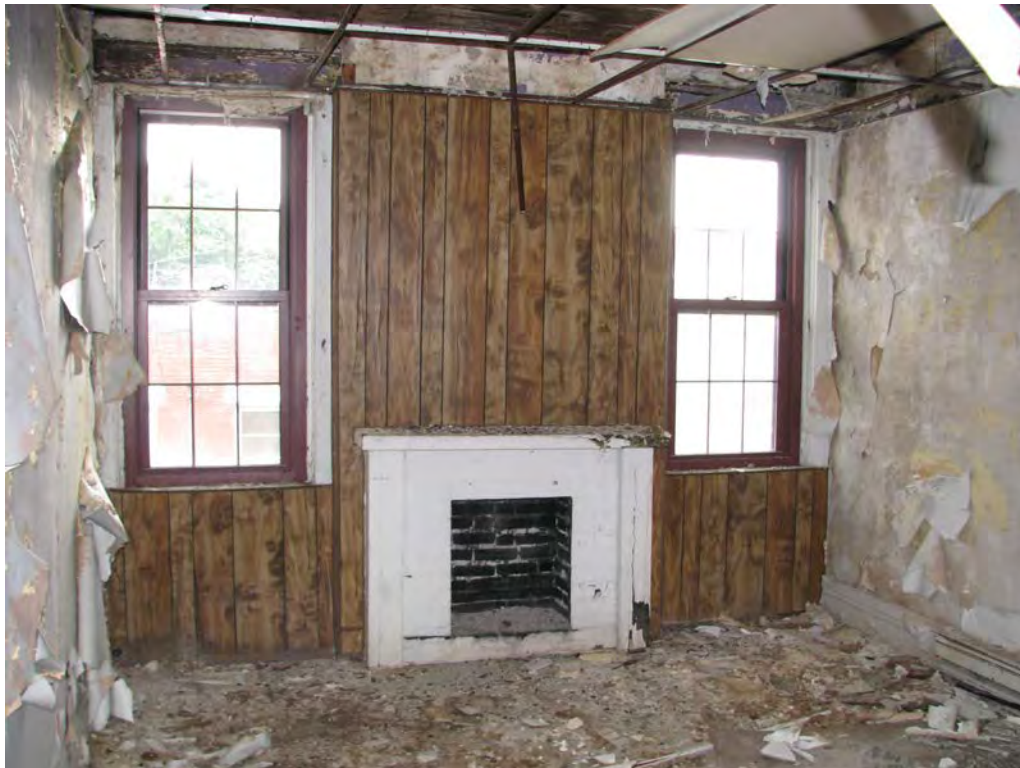
Photo 26. Third floor, rear apartment, looking east, showing that the fireplace and finishes have been altered from the original (P+A, 2018).
