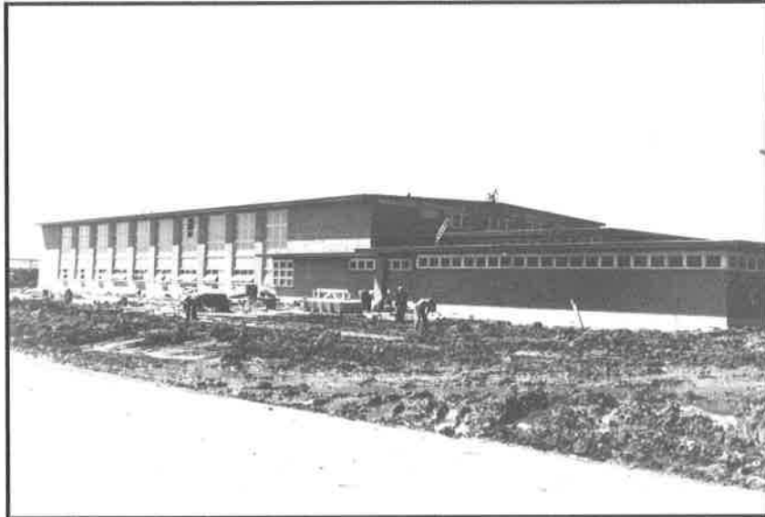
Figure 20 Swimming Pool Building under construction Official U.S. Navy Photograph (undated) (Courtesy of Wapello County Historical Society)
