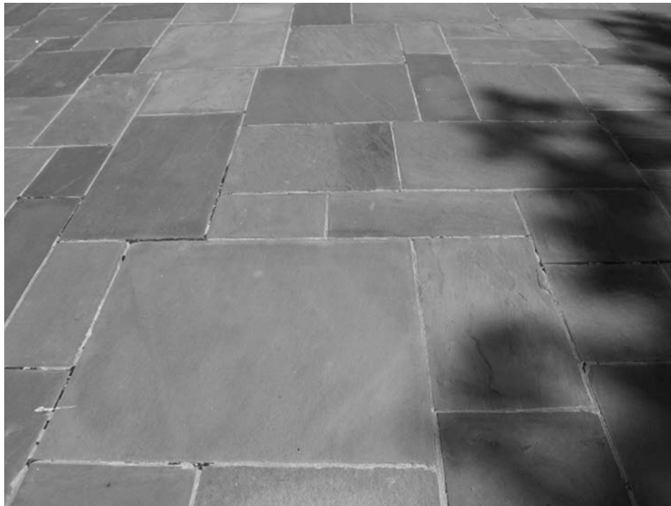
Photo 21. Detailed view of bluestone pavers located south of memorial shaft, looking north
