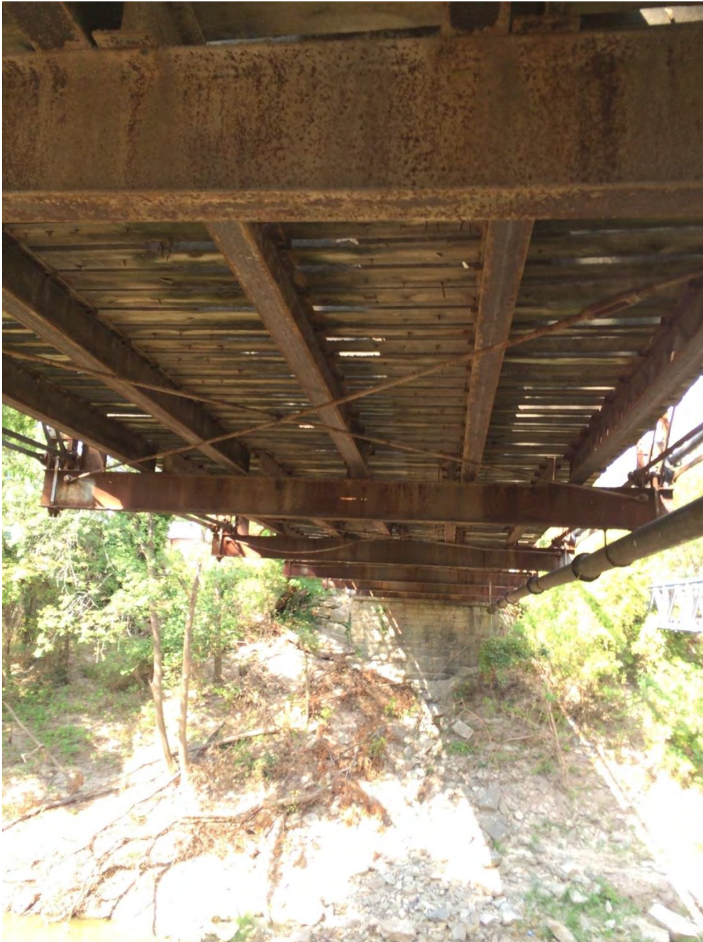
Photo 9: Floor beams and lateral bracing. Camera facing west. Photo by Linda Henderson, Texas Historical Commission
