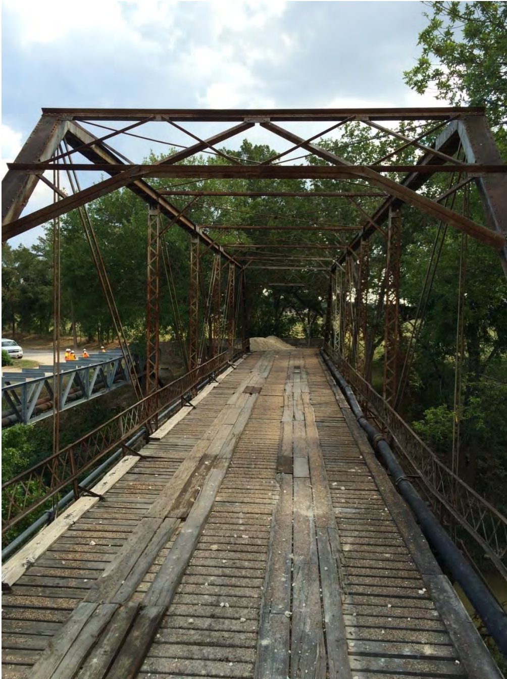
Photo 12: Deck, trusses, and latticed bracing from west portal. Camera facing east. Photo by Linda Henderson, Texas Historical Commission
