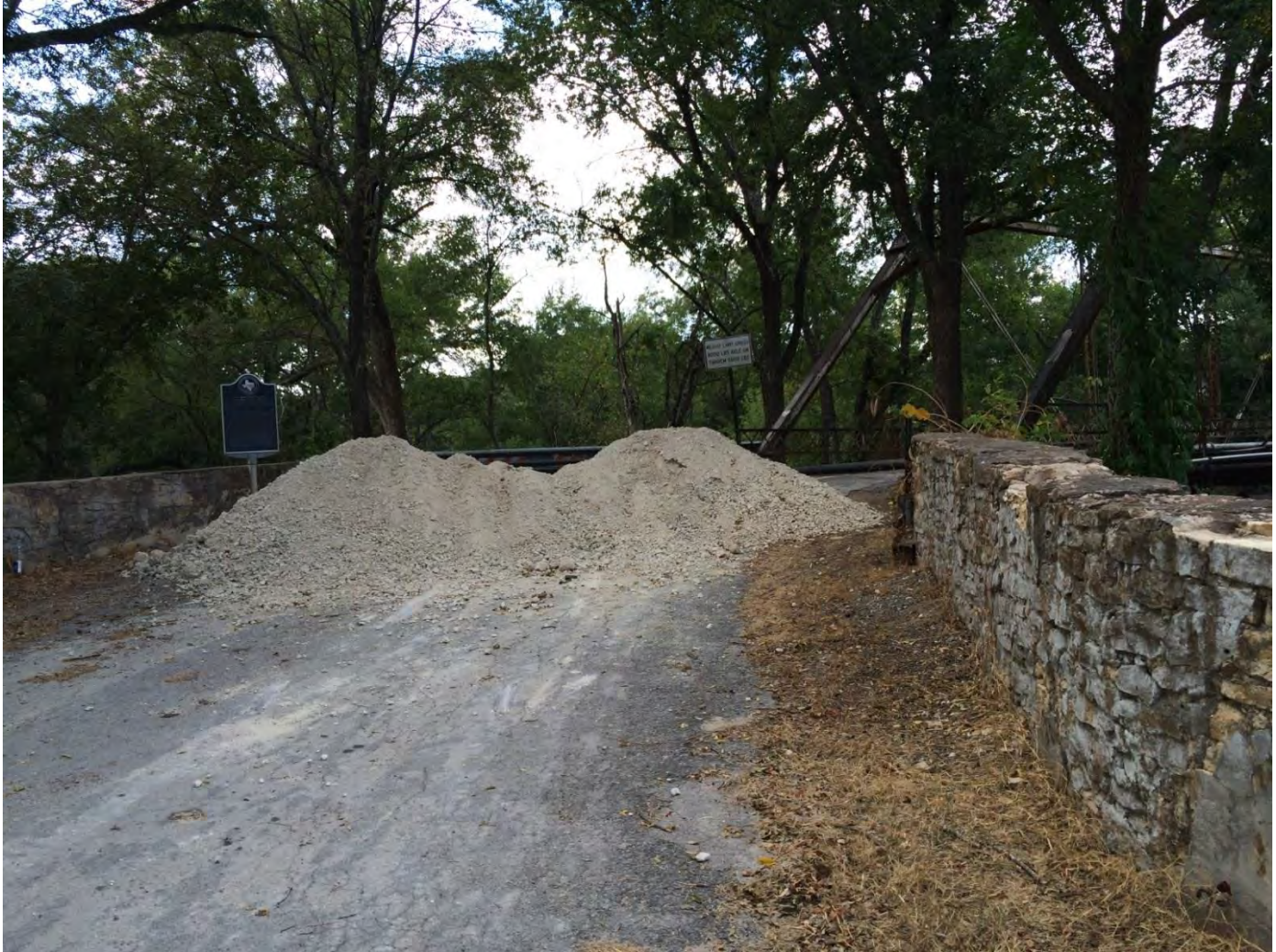
Photo 8: Stone masonry walls at east portal. Camera facing south. Photo by Linda Henderson, Texas Historical Commission
