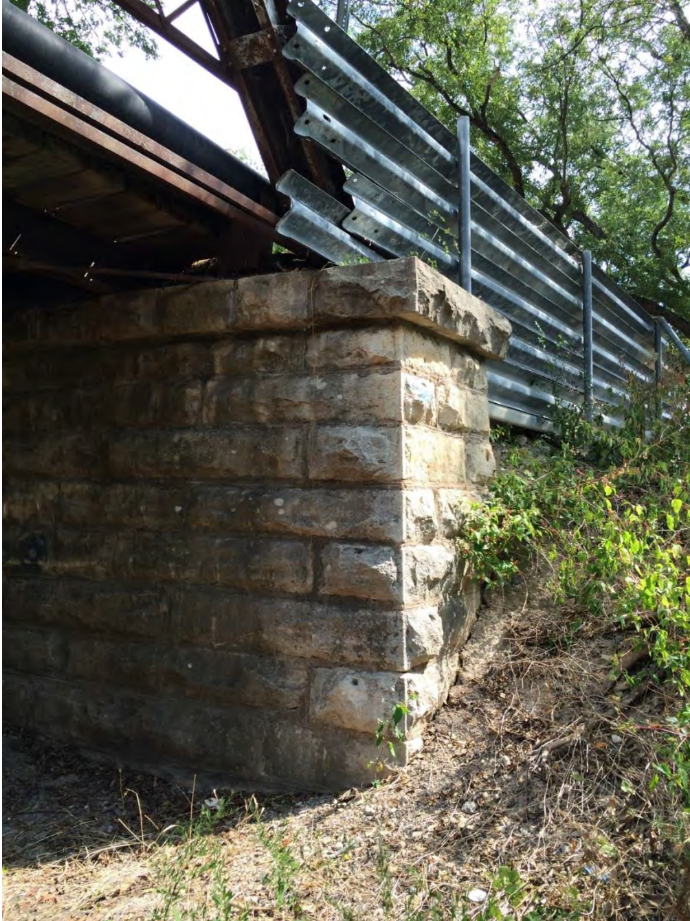
Photo 7: Stone masonry abutment. Camera facing east. Photo by Linda Henderson, Texas Historical Commission
