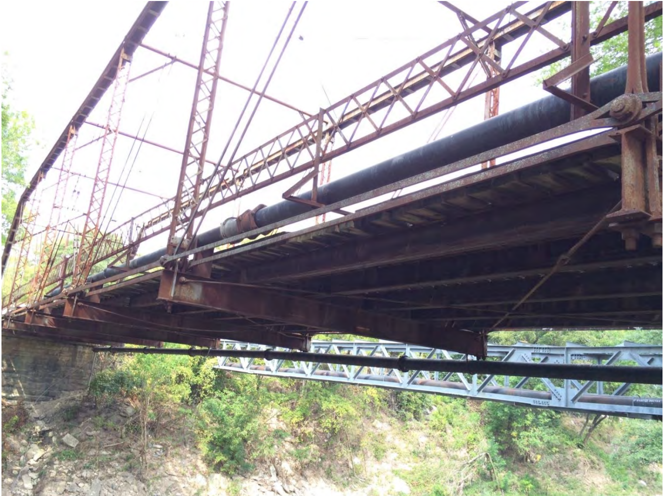
Photo 11: Utility pipe. Camera facing northwest. Photo by Linda Henderson, Texas Historical Commission
