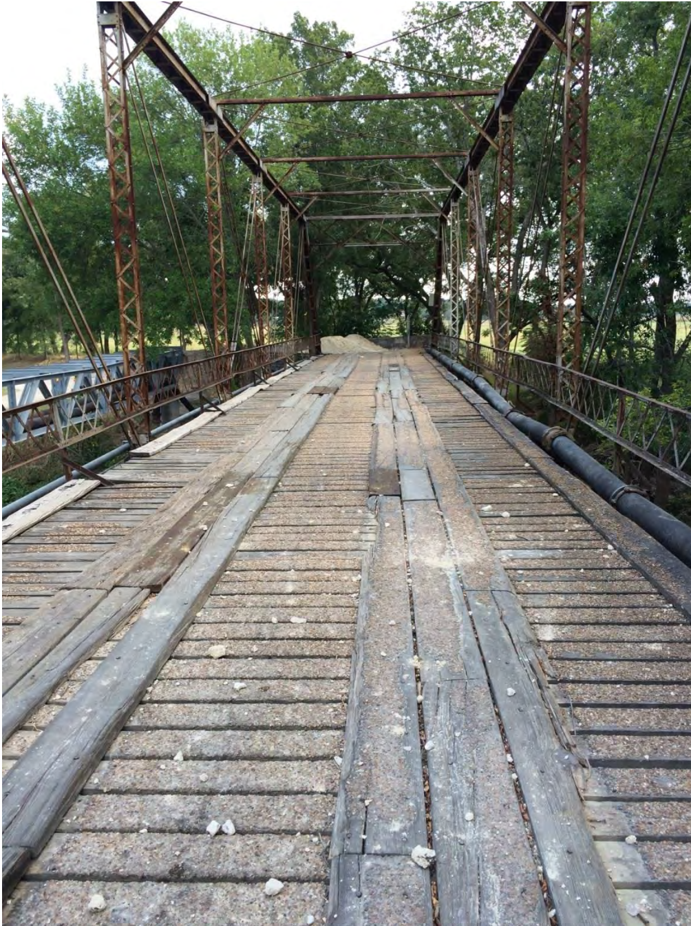
Photo 5: Deck and trusses from west portal. Camera facing east. Photo by Linda Henderson, Texas Historical Commission
