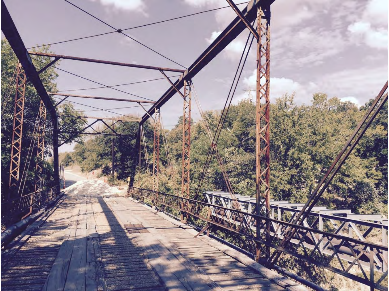
Photo 2: Deck and Pratt truss from east portal. Camera facing west. Photo by Rebekah Dobrasko, Texas Department of Transportation
