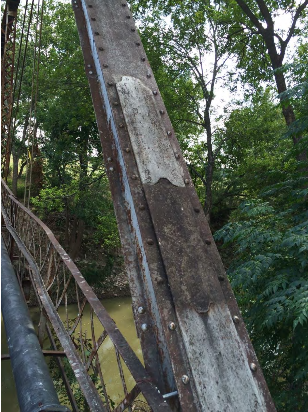
Photo 6: Inclined end post on south side. Camera facing east. Photo by Linda Henderson, Texas Historical Commission
