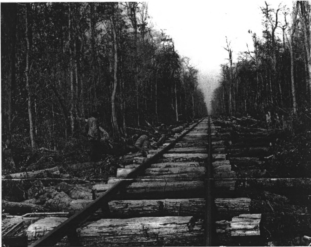
Main line in Okefenokee between the Swamp's edge and Cravens Hammock constructed with a pile driver - 10" caps (hewn 2 sides) fastened to piles with \frac{3}{8} " iron drift bolts - 7 bents to 39-foot rail (Hopkins, 45 Years with the Okefenokee Swamp , 1947; RG-50-2-33, S.W. McCallie, March 1915, Georgia Department of Archives and History, Atlanta, Georgia).
