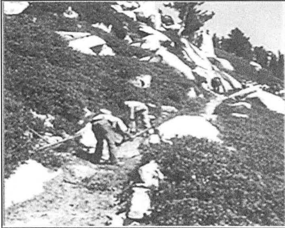
Photograph # HP9 Looking Northeast at Trail Repair Work Date: 1957 August 8 Source: CA State Museum Accession # 090-23933
