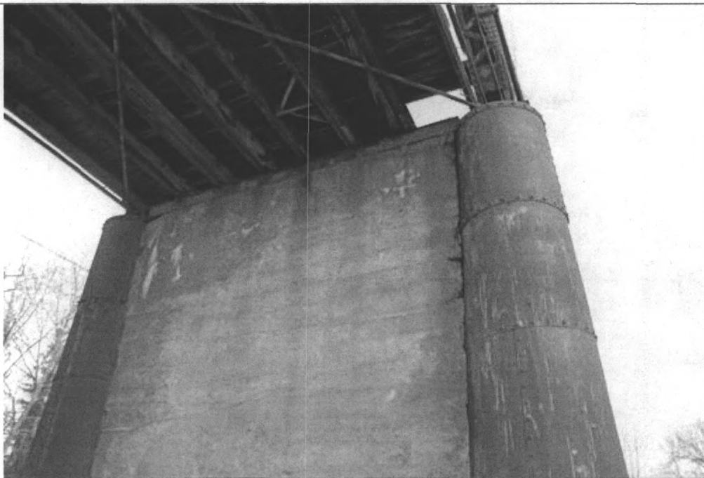
Photo 0005. Detail of south abutment of Flathead River Bridge. View to the southeast.
