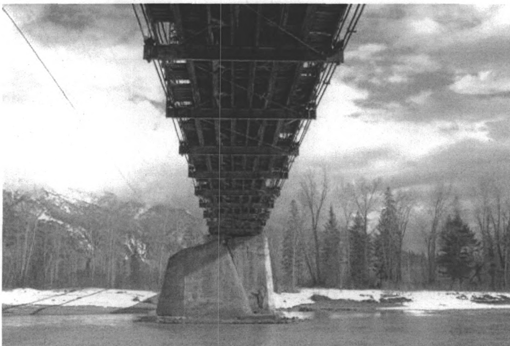
Photo 0006. Concrete pier and understructure of Flathead River Bridge. View to the south.
