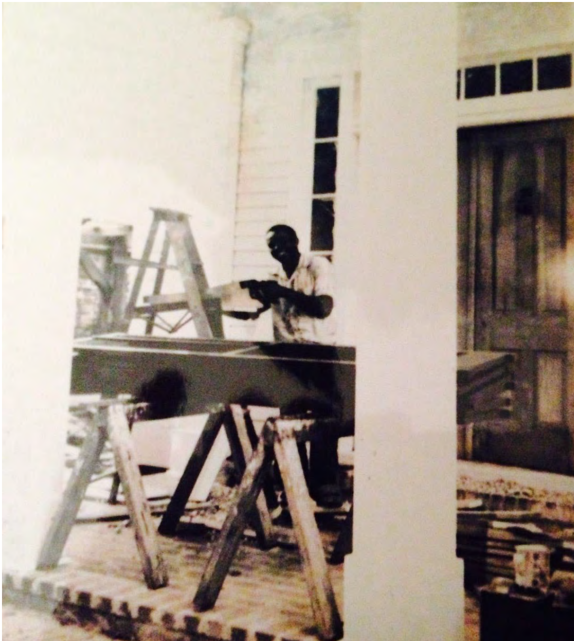
Figure 1: Nathaniel Guydon working on the construction of the Moore-Jacobs House Chapel, c.1950.
