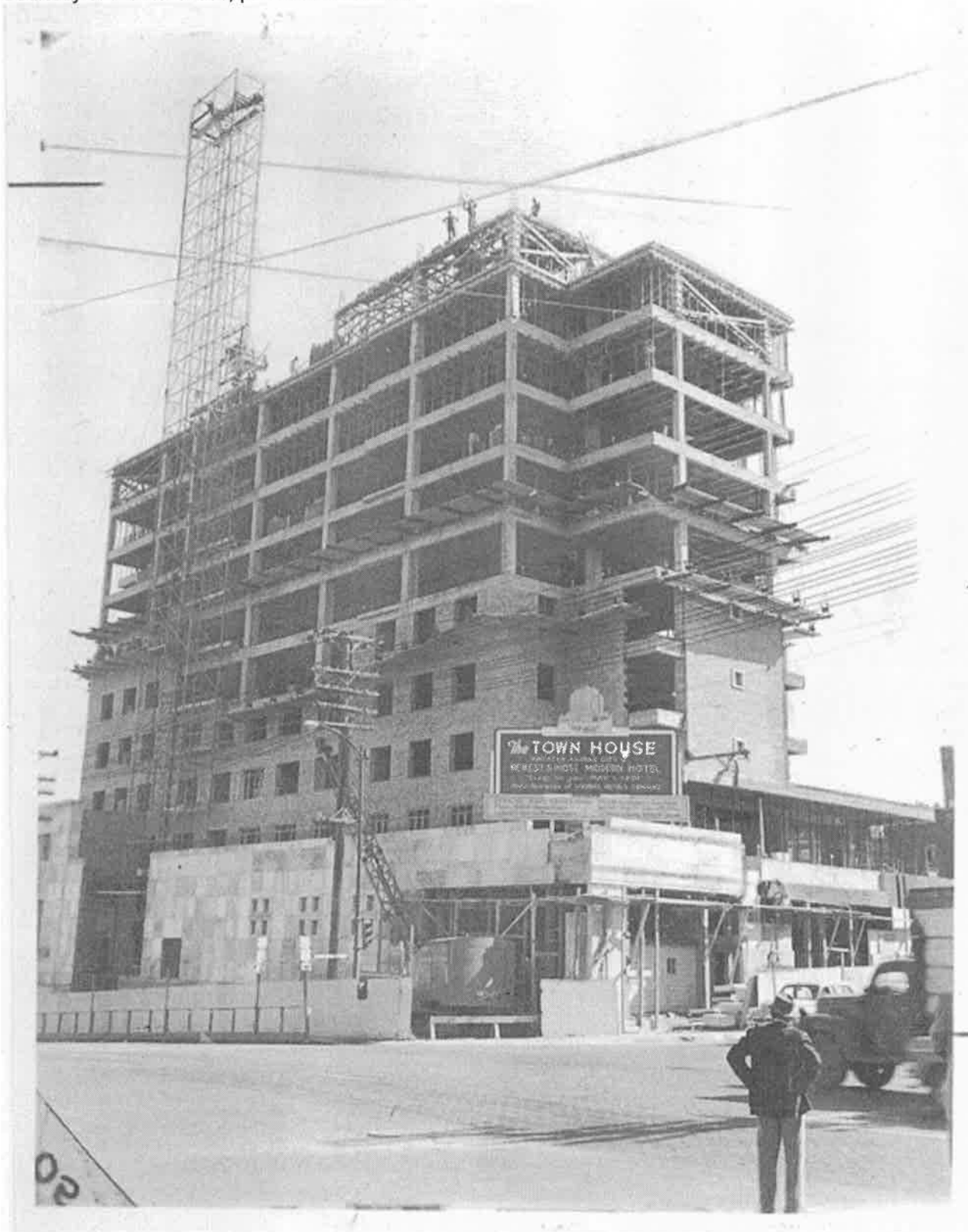
Figure 5. Town House Hotel during construction, c. 1950. Courtesy of Monte Gross, personal collection.
