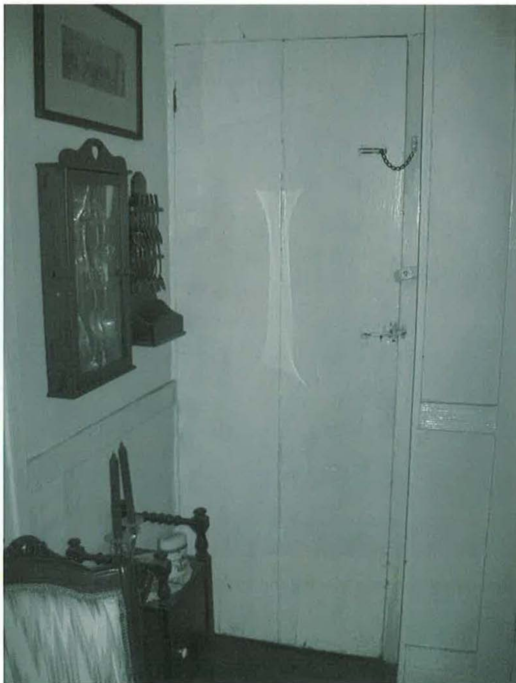
Interior of central hall, showing cellar access door details. Camera facing southeast. Photograph 10 of 20.
