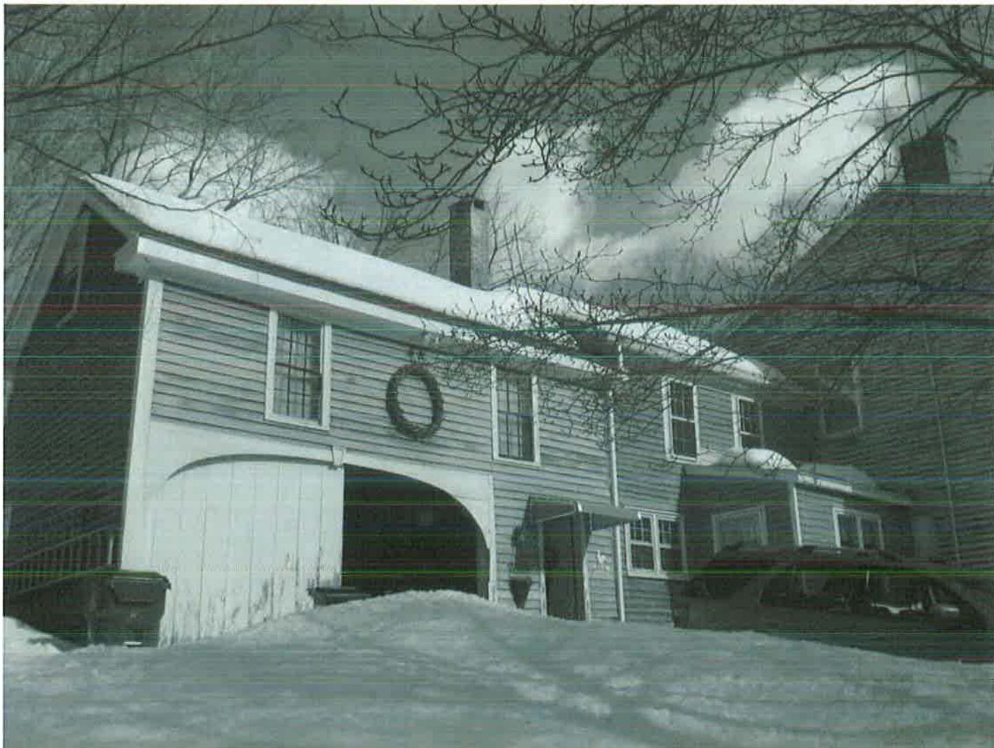
South (front) and west (side) elevations of side ell, showing window, window surround, trim, and cornice details.
