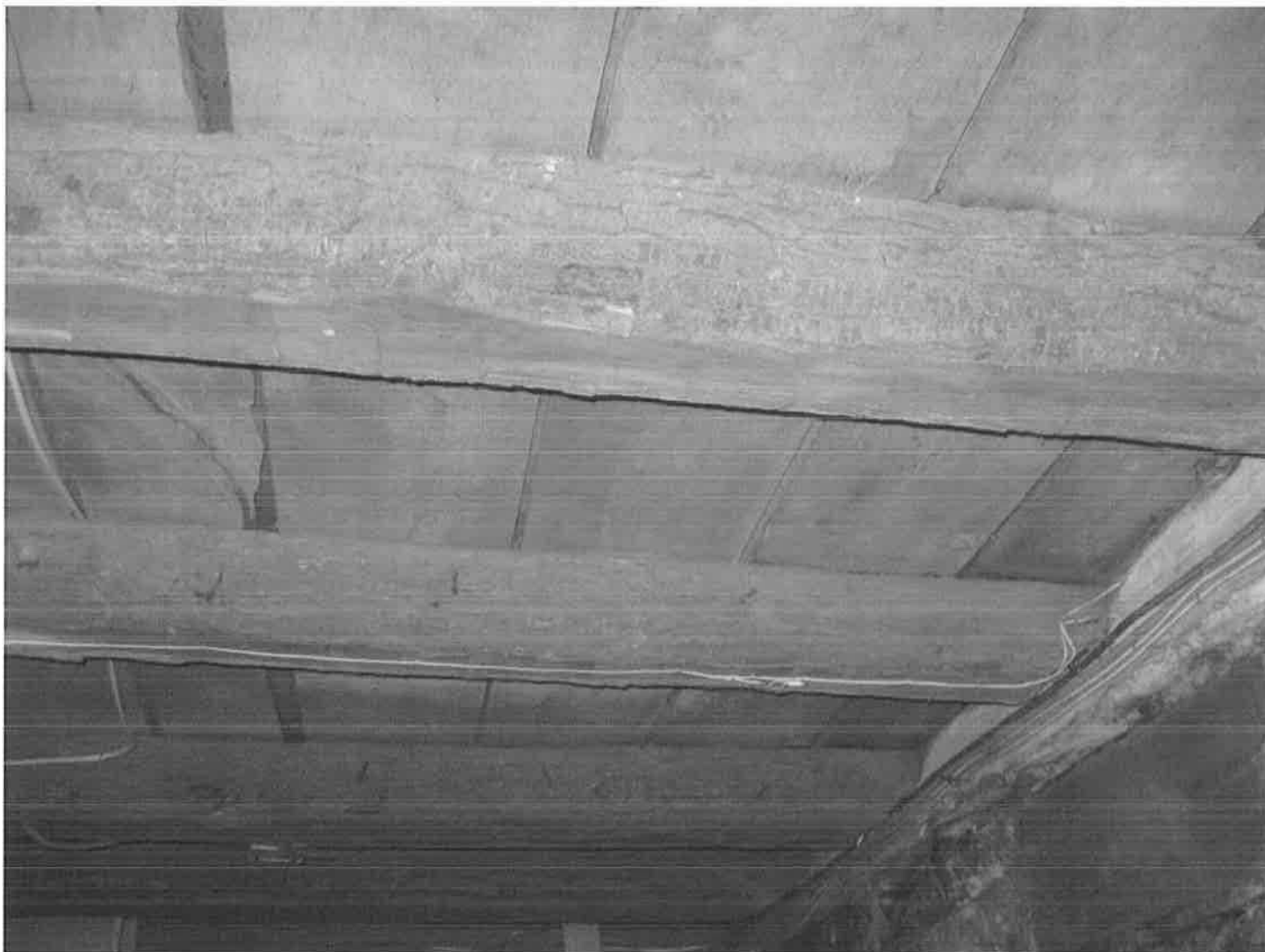
Interior of cellar, showing first-floor framing and floorboard details. Camera facing east. Photograph 11 of 20.
