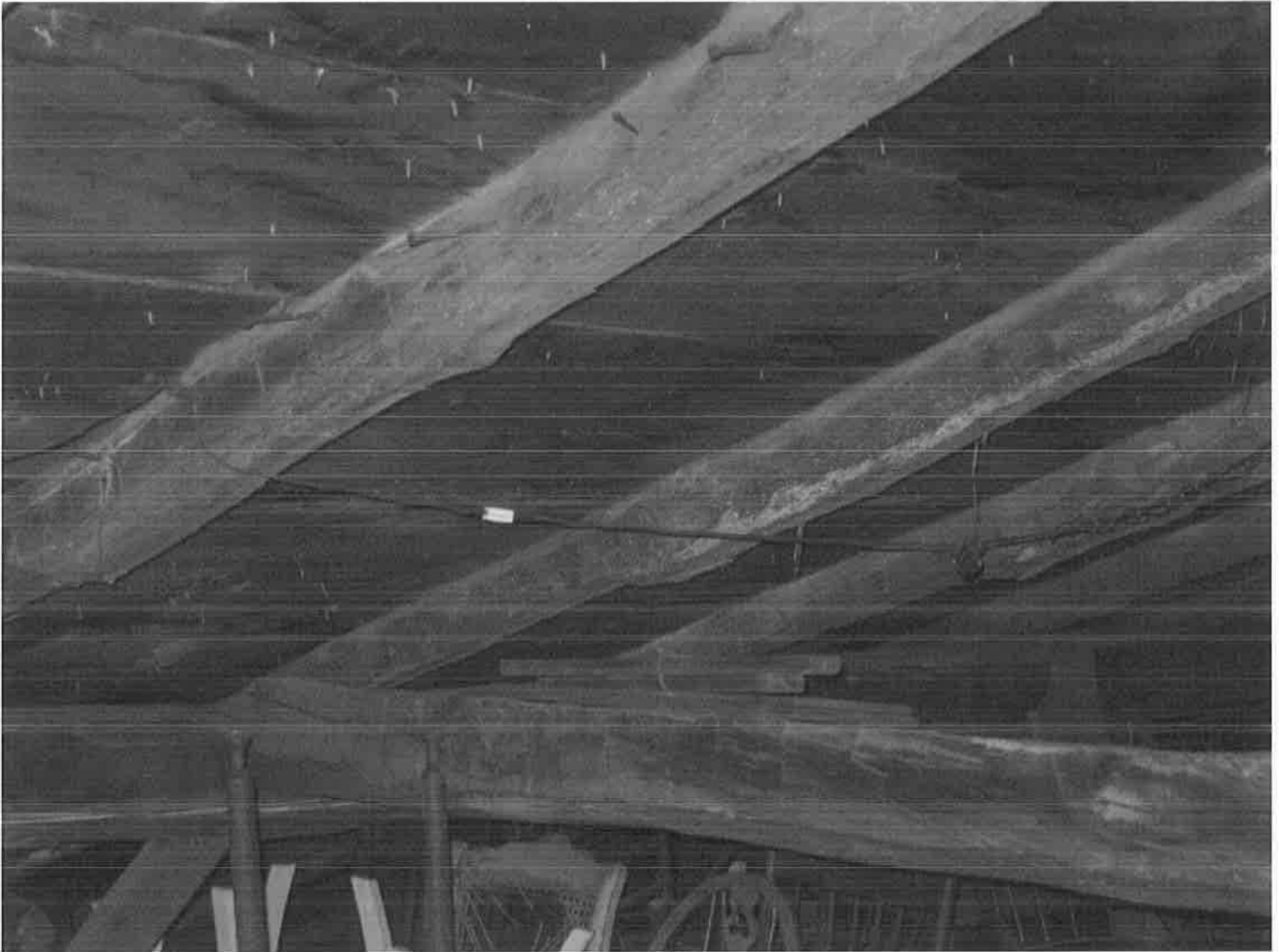
Interior of attic, showing rafter, purlin, brace, and roof sheathing details. Camera facing southwest. Photograph 19 of 20.
