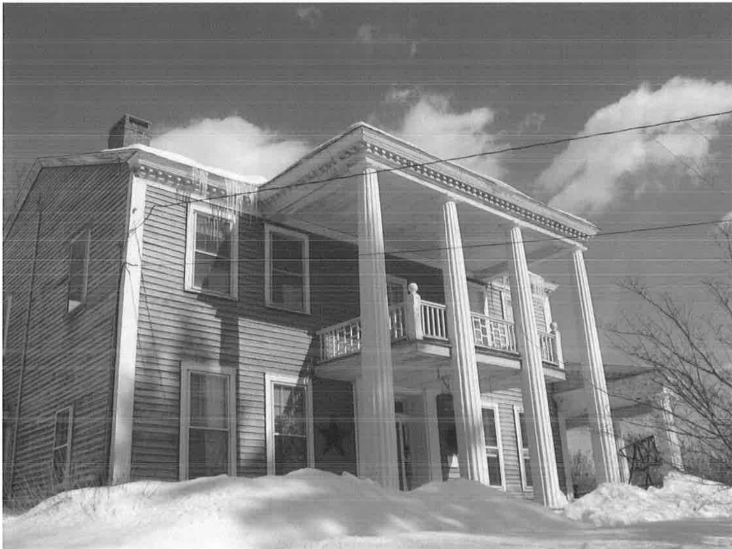
South (front) and west (side) elevations of house from Spoonville Road, showing window, window surround, trim, cornice, and porch details. Camera facing northeast. Photograph 3 of 20.
