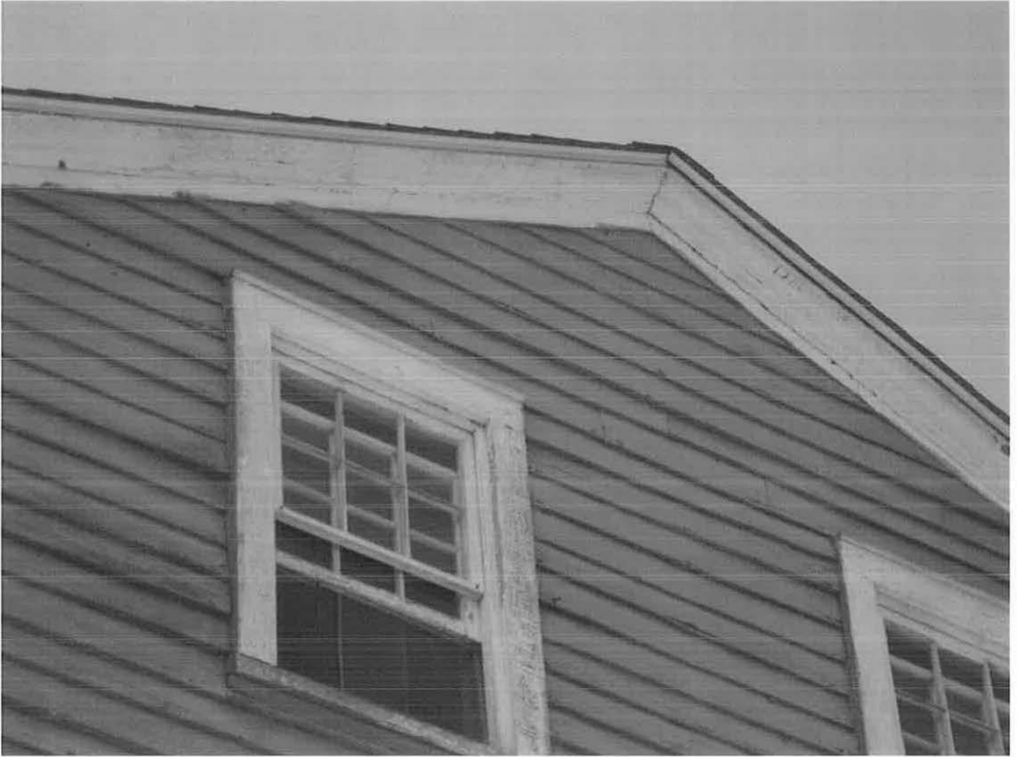
East (side) gable end of house from the "Old County Highway", showing molded rakeboards. Camera facing northwest. Photograph 5 of 20.
