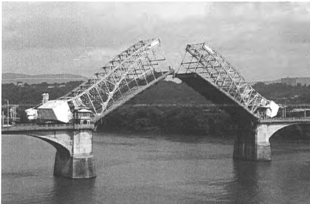
Figure 5. Market Street Bridge, no date, during routine inspection. From Tennessee's Survey Report for Historic Bridges
