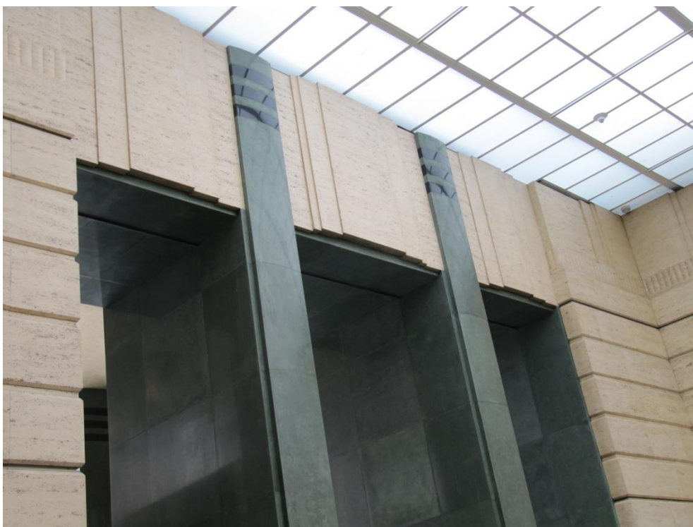
018 Interior view of the west wall and skylight in the Garden Court
