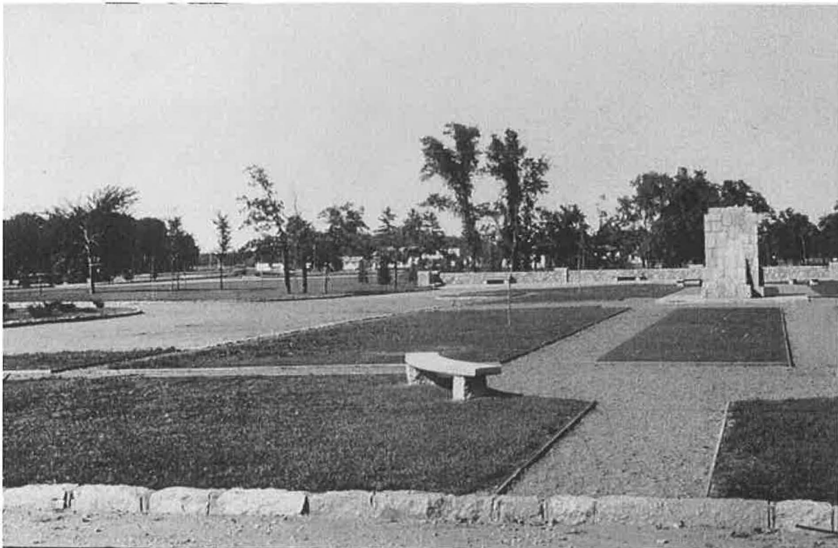
Figure 6. The concourse nearing completion. The central island has a stone flagpole base approached by a grid of gravel walkways. The granite curbing and curved benches have been built, but the metal flagpole has not yet been installed and the shrubs have not been planted (photo by Minnesota Dept. of Highways, probably summer or fall 1939, camera facing north, Dept. of Transportation Collection, Minnesota Historical Society).
