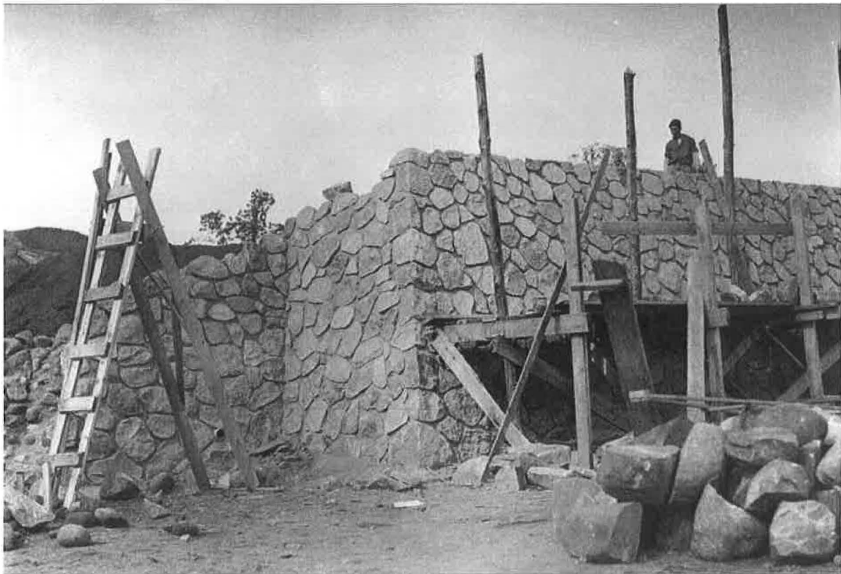
Figure 4. CCC workers building the stone overlook wall. Construction could occur on dry land because drought in the 1930s had lowered the level of the lake. During years of normal rainfall and lake levels, the water laps at the base of the stonework (photo by Minnesota Dept. of Highways, probably summer 1937, camera facing northwest, Dept. of Transportation Collection, Minnesota Historical Society).
