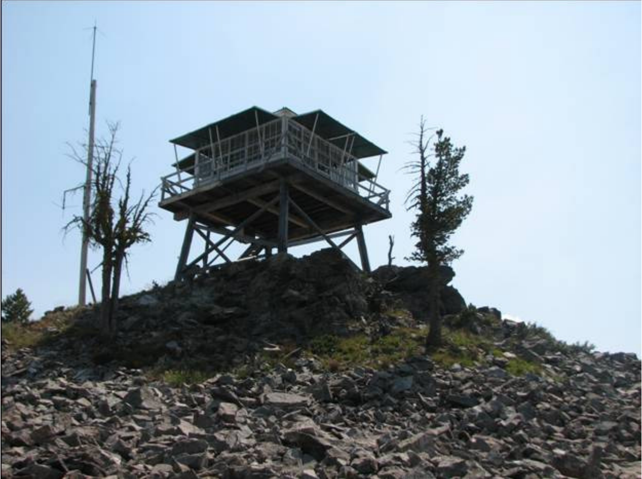
MT_RavalliCounty_MedicinePointLookout_0001. Looking east-east to the north and west walls of the lookout. The antenna pole is shown at the northeast corner of the lookout.
