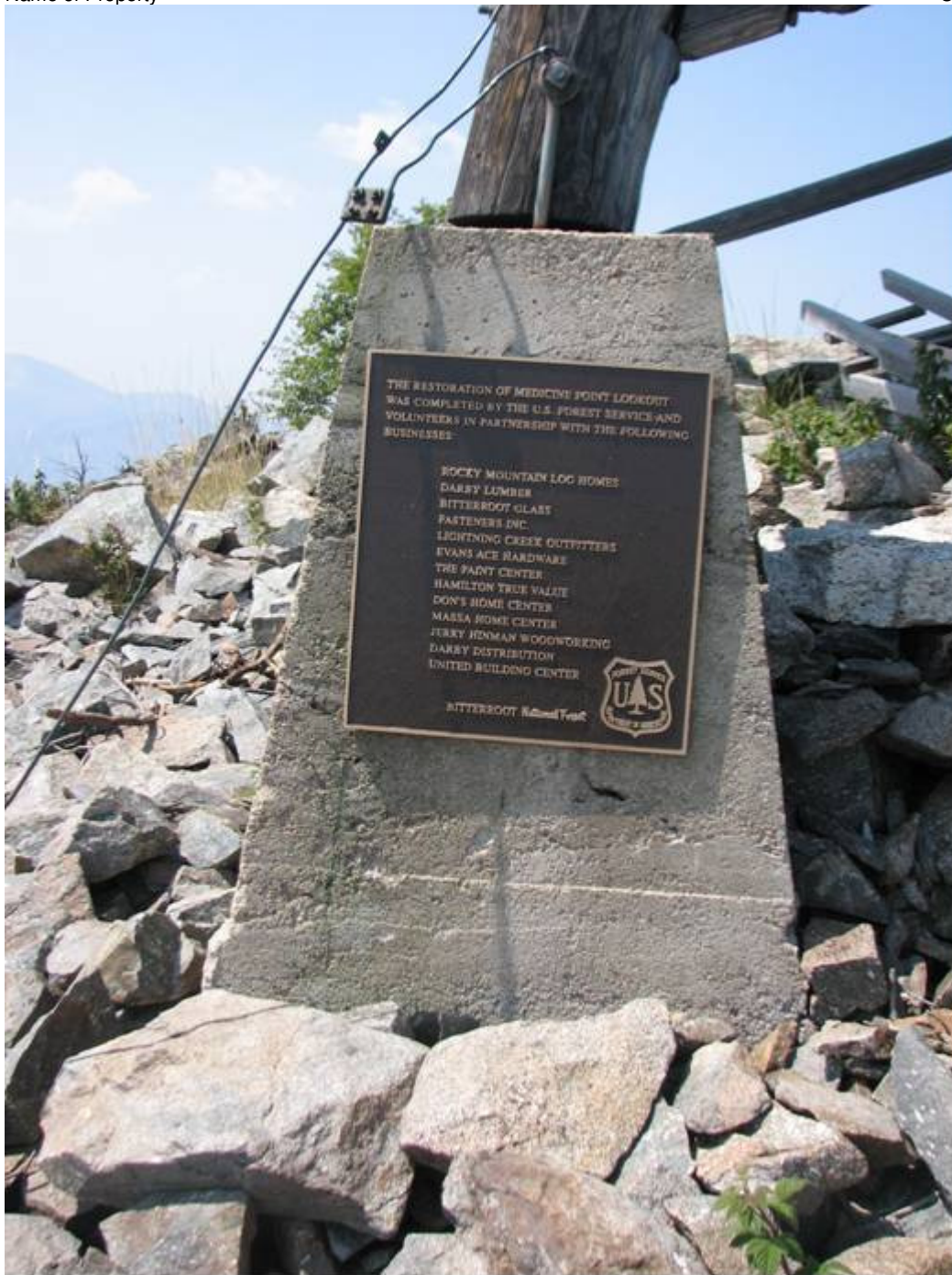
MT_ RavalliCounty_MedicinePointLookout_0005. Detail of the battered concrete pier at the southeast corner of the look with commemorative plaque.
