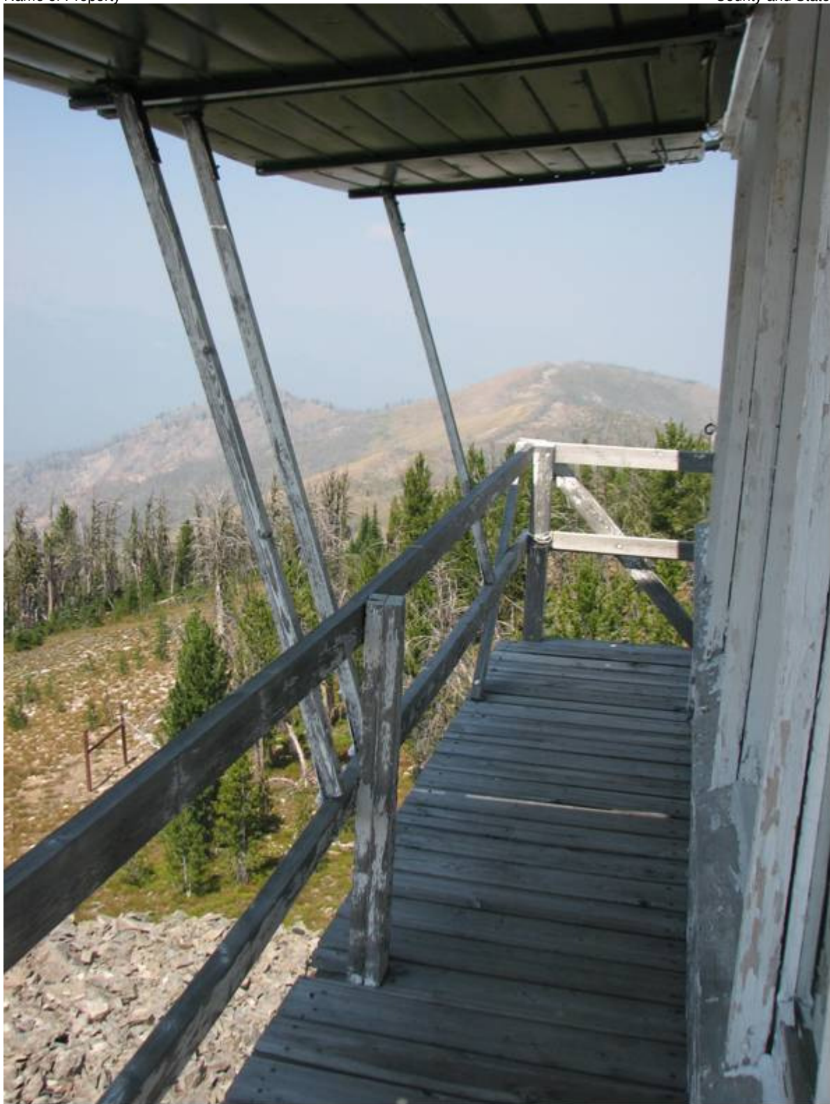
MT_ RavalliCounty_MedicinePointLookout_0006. Looking north along the catwalk on the west wall of the lookout cab.
