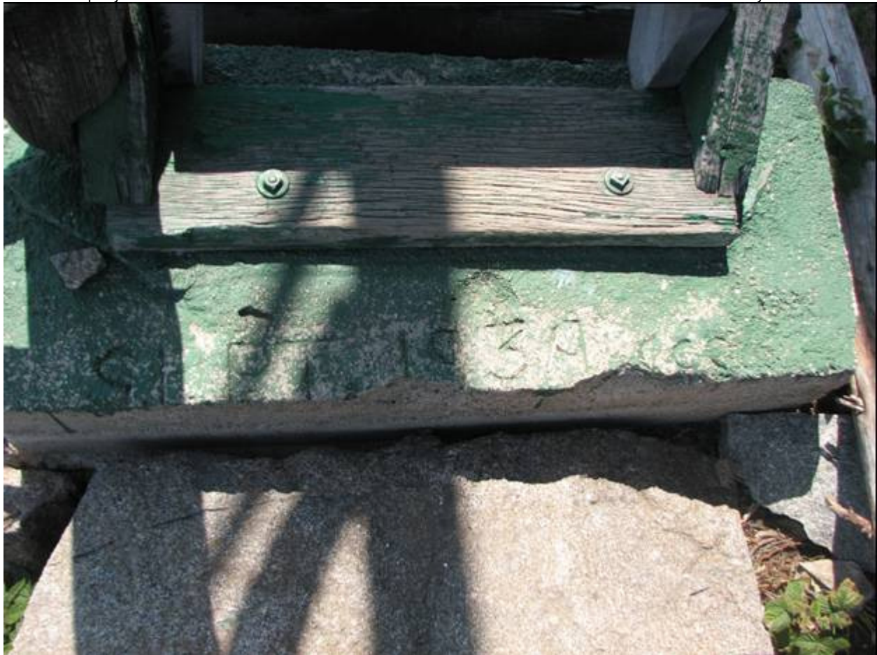
MT_RavalliCounty_MedicinePointLookout_0004. Detail: concrete footing at base of stair impressed with "SEPT 1939 ccc"
