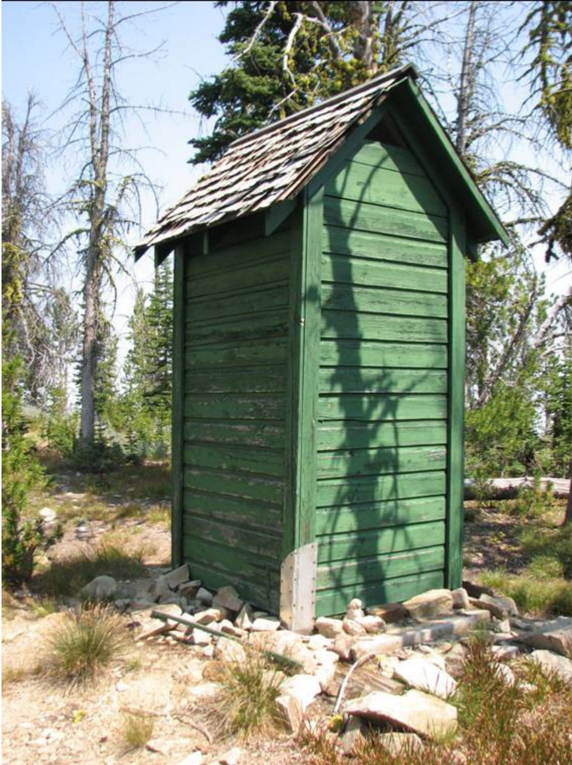
MT_ RavalliCounty_MedicinePointLookout_0012. Looking northeast to the west and south walls of the outhouse.
