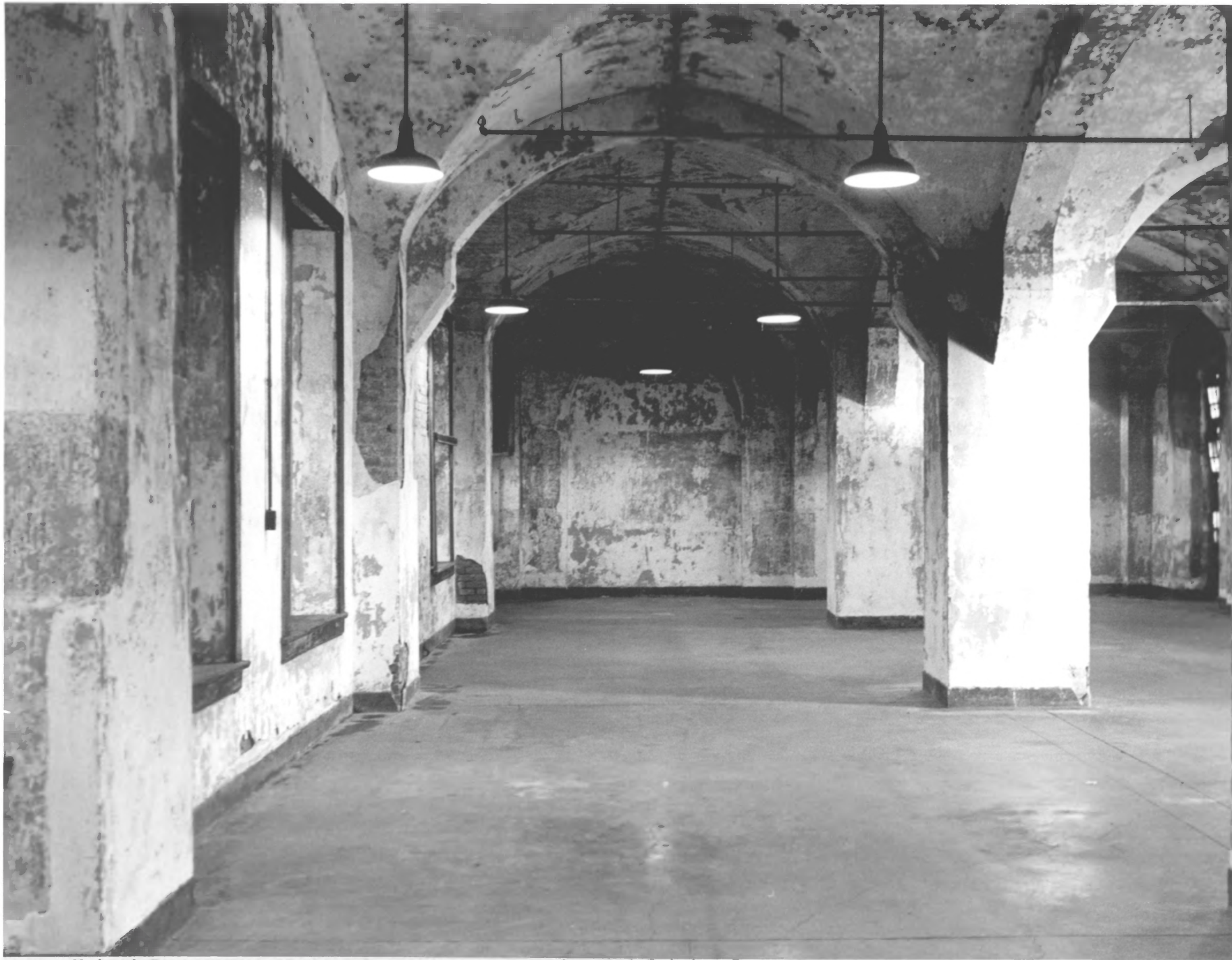
United States Branch Mint, New Orleans--Counting and Coining Room, Principal level. NPS Photo 1974
