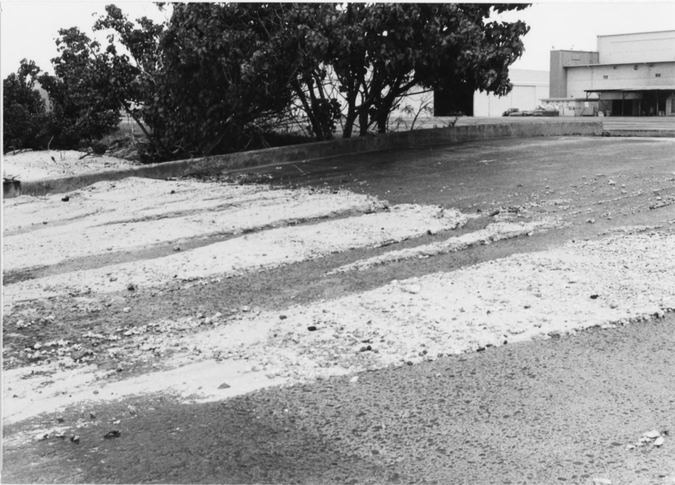
Seaplane ramp no. 1 which leads into Kaneohe Bay. Former Kaneohe Naval Air Station is now a Marine Corps air station.
