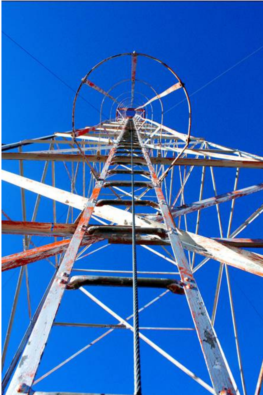
Photo #0004: MacDonald Pass Airway Beacon. View to top of beacon from the south side of tower. Photo date: April 1, 2013.
