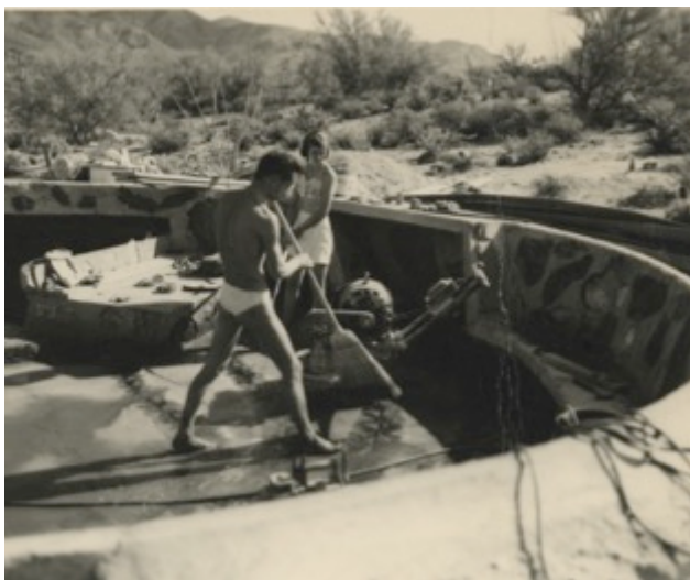
Figure 8c. Photographs of the Dome House under construction. Paolo Soleri and his wife Colly are in most images. Courtesy of Kristine Soleri-Timm.
