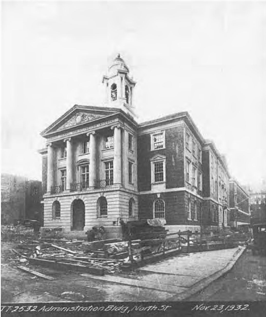
Figure 2: 1932 View during construction of the primary (south) elevation of the Traffic Tunnel Administration Building, with views of the east elevations of the Boston Police Station Number One and Boston Printing Department Buildings (source: UMASS Boston Archives and Special Collections).
