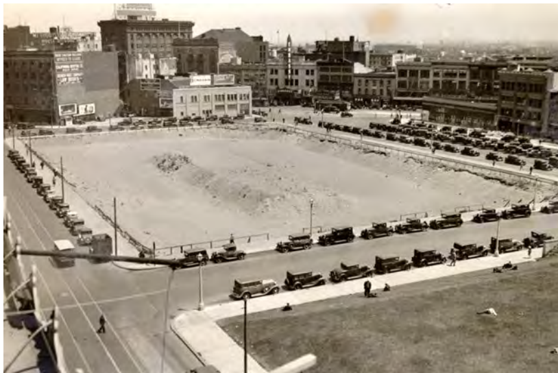
Figure B. Site excavation nearing completion, July 1933 (San Francisco History Center, San Francisco Public Library)
