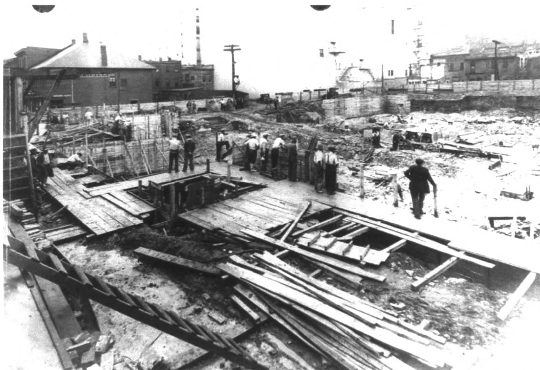
Figure 21 Excavation of the Federal Building's basement appears to have been well "supervised" in the spring of 1932. This view looks southwest from the corner of Perry and 4 th Streets. The white building with the fire escape stairs in the center background is the alley side of the RKO Orpheum Theater (now Adler Theater). The hipped roof building in the far left is a part of the Windsor Hotel (nonextant). (Collection of the General Services Administration, Kansas City, Missouri)
