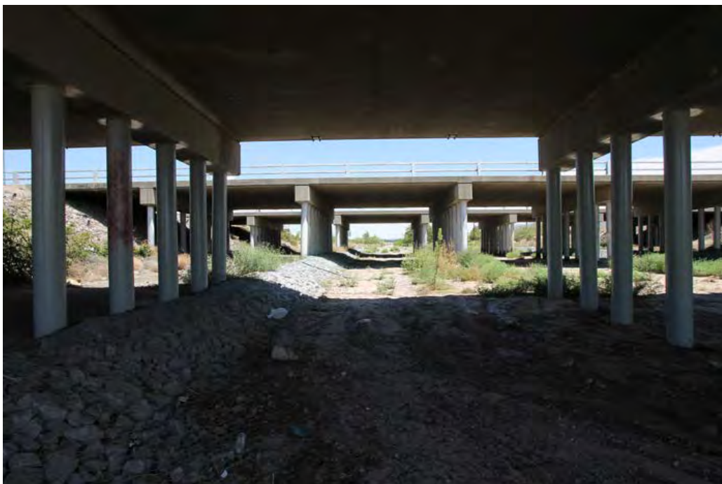
27 of 56. Tortugas Arroyo with Interstate 10 overpasses, photographer facing northeast. (Not in National Register boundary.)
