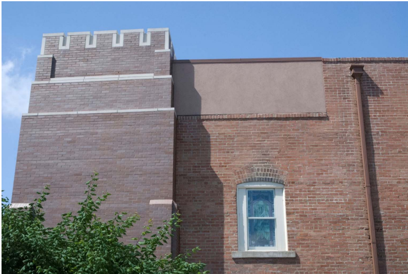
Photo 20: Rear (Northeast) Elevation, Detail, Smoke Damage, camera facing southwest.
