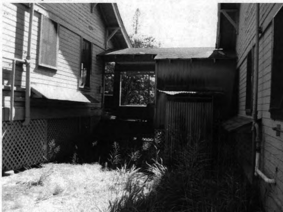
FBMH-001-006. Fred Baldwin Memorial Home, Connecting Lanai between Buildings 001 and 002, Looking Southwest.
