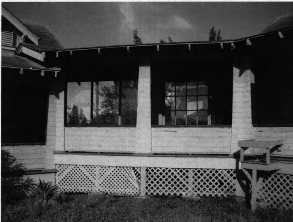
FBMH-002-004. Fred Baldwin Memorial Home, Connecting Lanai between Buildings 002 and 003, Looking Northeast.
