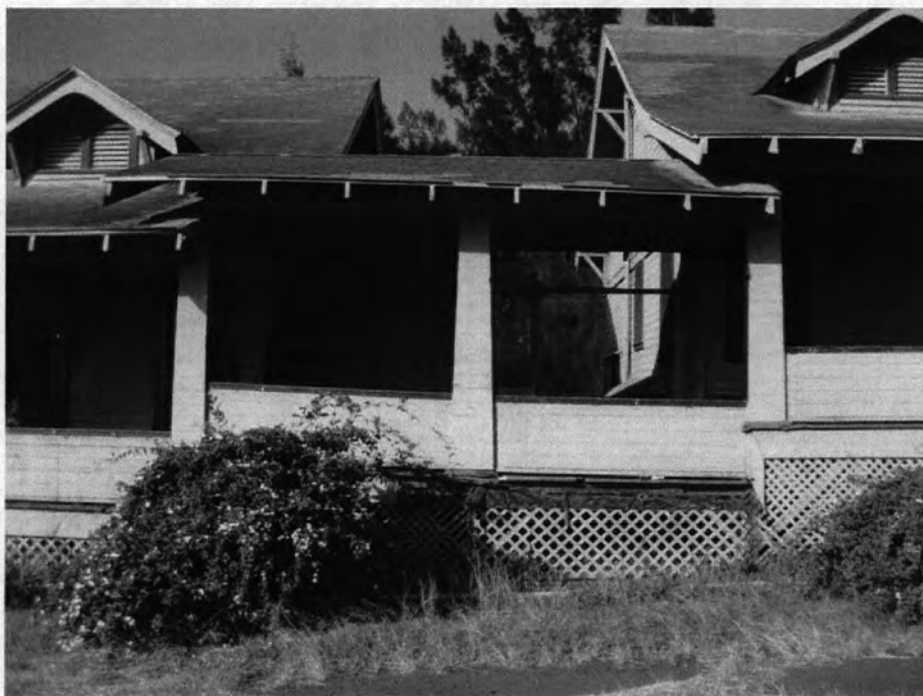
FBMH-001-005. Fred Baldwin Memorial Home, Connecting Lanai between Buildings 001 and 002, Looking Northeast.
