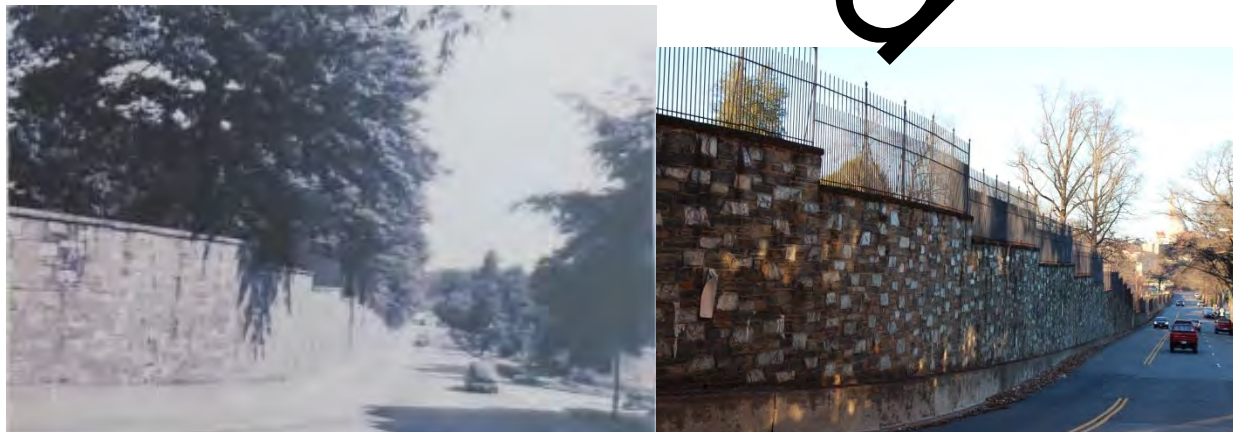
Historic and Current Photos of Lincoln Retaining Wall Source: Glenwood Cemetery Archives; EHT Traceries
