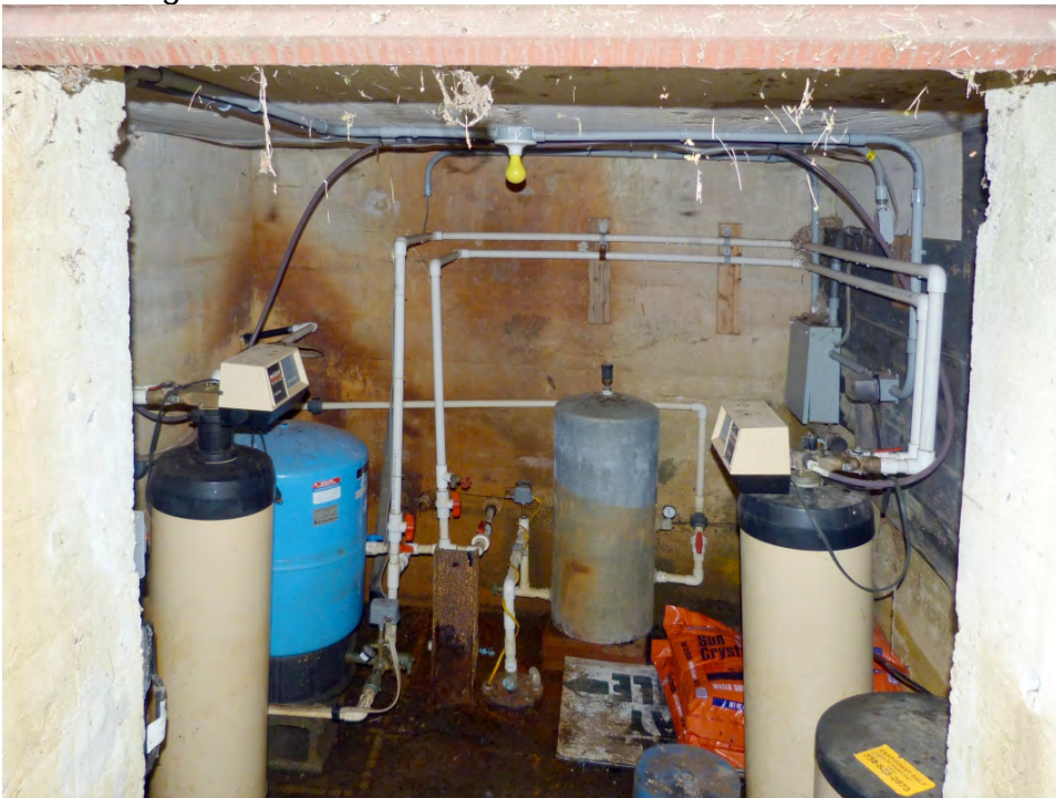
NJ_BURLINGTON_RIDGWAY, HOUSE, WILLIAM_0053 View facing south in the pump house.
