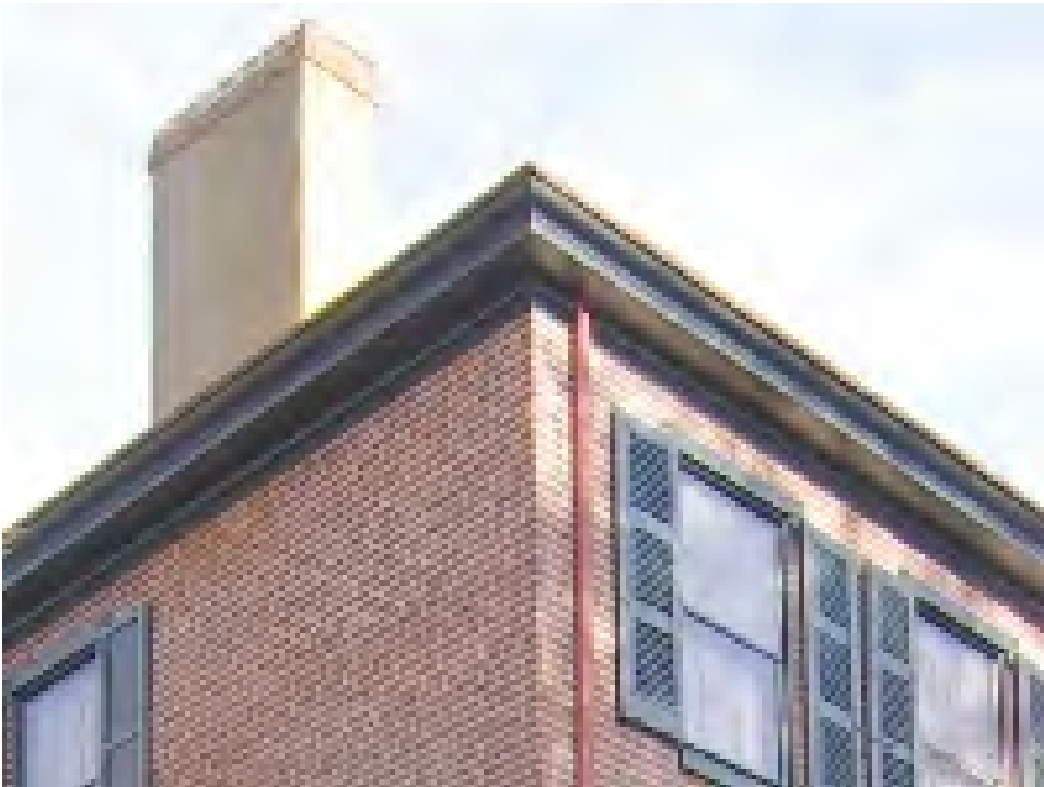
NJ_BURLINGTON_RIDGWAY, HOUSE, WILLIAM_0014 Detail facing northeast showing the southwest cornice and a chimney.
