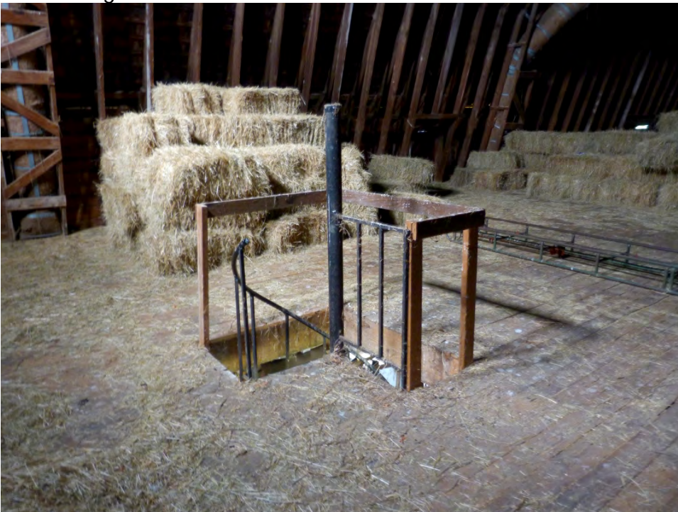
NJ_BURLINGTON_RIDGWAY, HOUSE, WILLIAM_0051 View facing northwest in the second floor of the barn.
