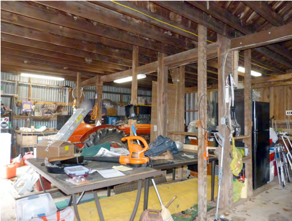
NJ_BURLINGTON_RIDGWAY, HOUSE, WILLIAM_0058 View facing northwest showing the interior of the corn crib.
