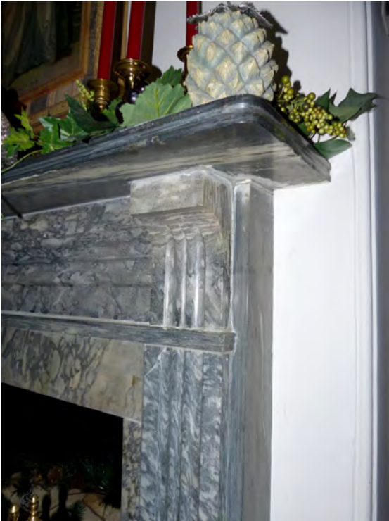
NJ_BURLINGTON_RIDGWAY, HOUSE, WILLIAM_0026 Detail showing the carved marble fireplace surround in the northwest parlor.
