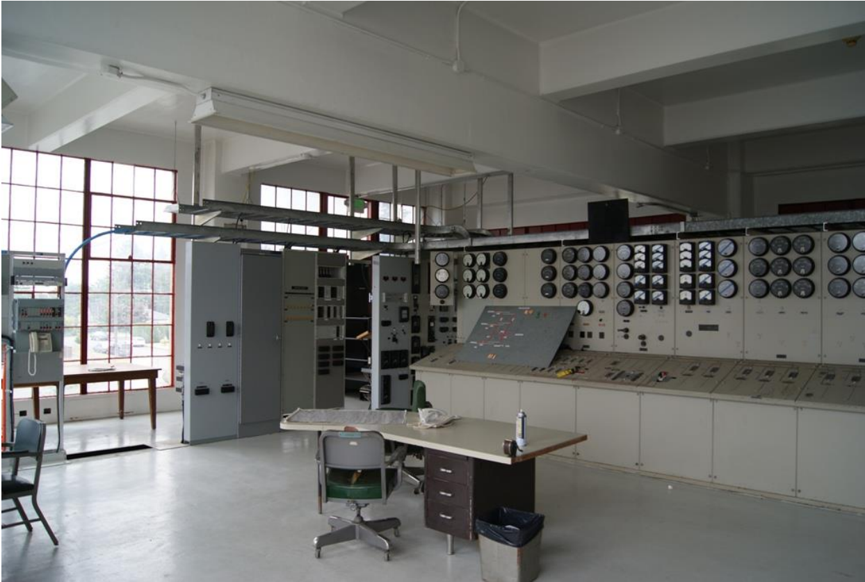
Photo 11 of 17. WA_PierceCounty_CushmanSubstation_0011. Former control room at Cushman Substation. The equipment is modern, though the room retains its original function.
