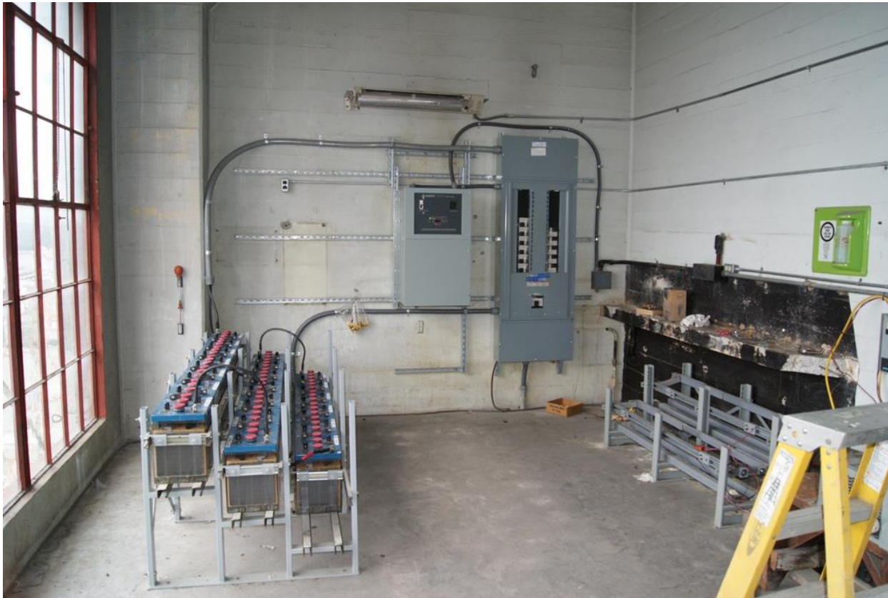
Photo 13 of 17. WA_PierceCounty_CushmanSubstation_0013. Battery room at Cushman Substation.
