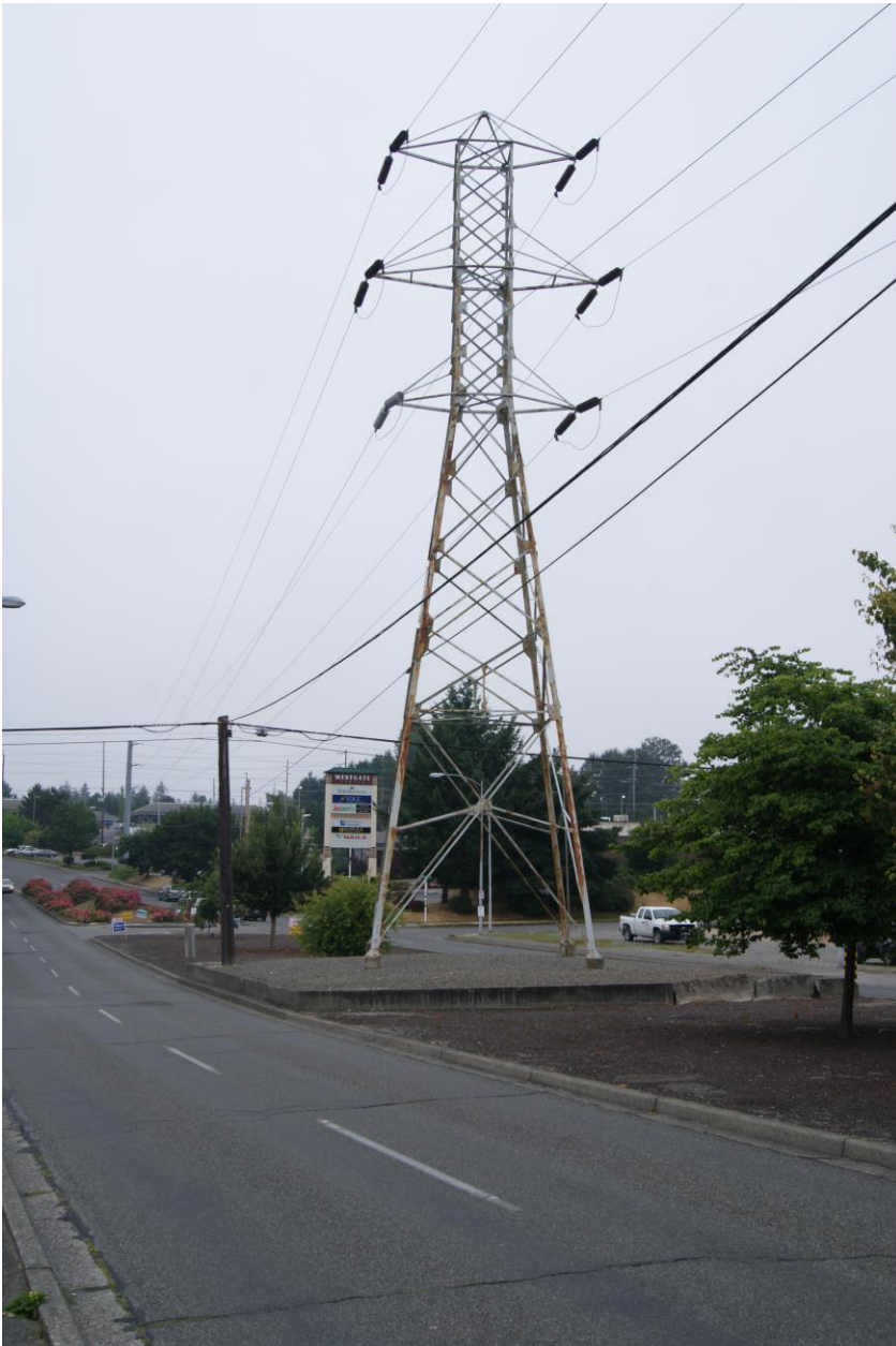
Photo 16 of 17. WA_Pierce County_Cushman Substation_0016. Typical Tower as traverses down N 21 st St.
