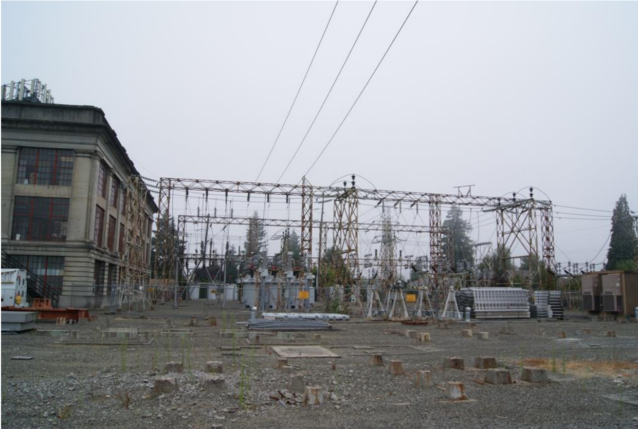
Photo 6 of 17. WA_PierceCounty_CushmanSubstation_0006. Viewing west to the exterior, modern switchyard (noncontributing) at Cushman Substation.
