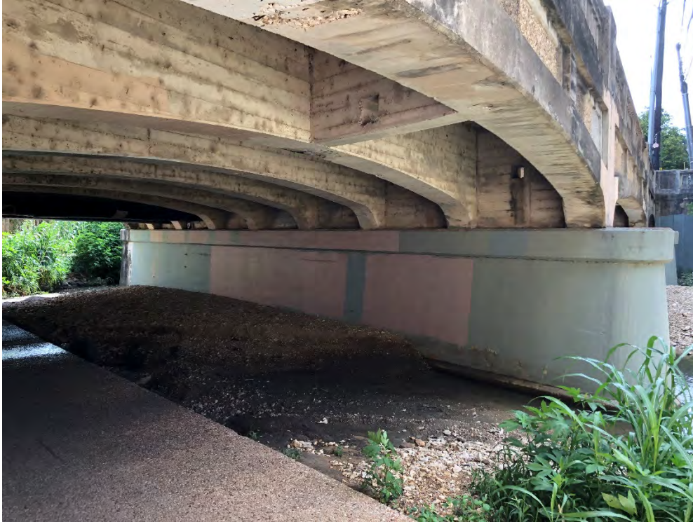
Photo 3: Concrete girders under bridge showing imprint of wooden forms used in construction. South side. View northeast.
