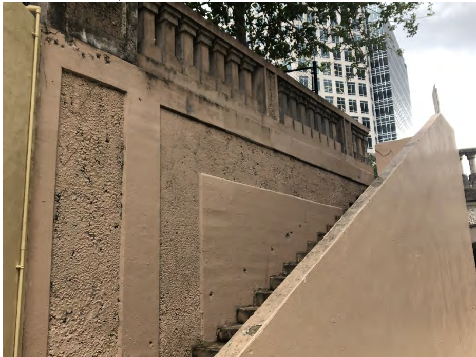
Photo 8: Staircase to access Shoal Creek trail. Southwest corner of the bridge. View northwest. (Photographed by Rebekah Dobrasko, October 2018).
