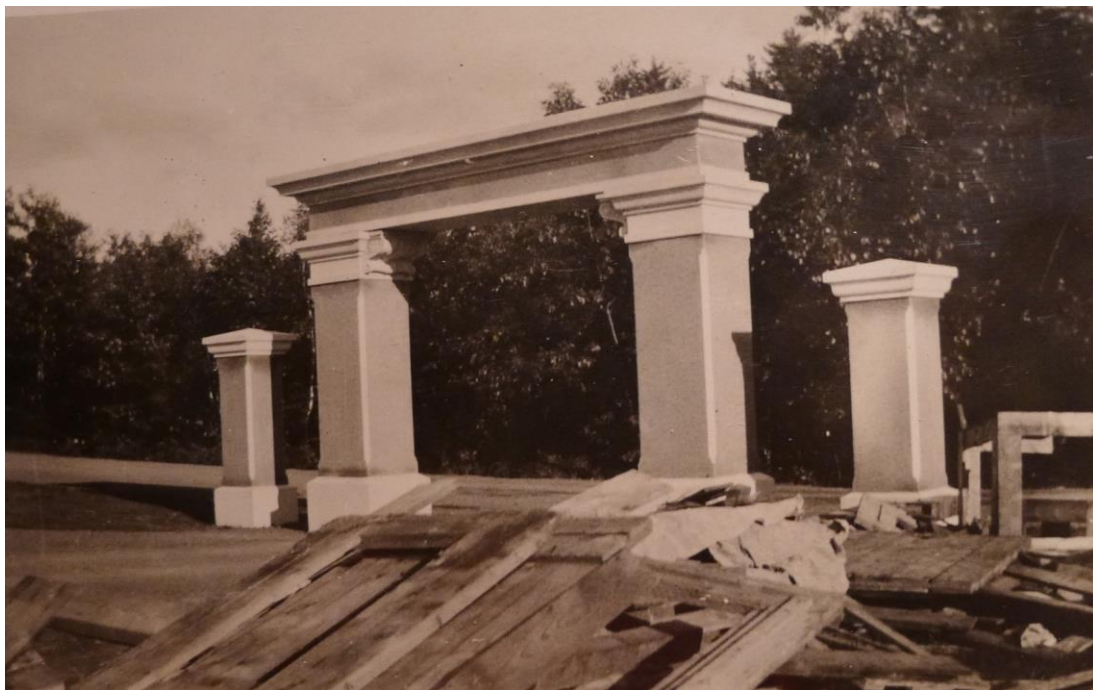
FIGURE 4 South Gate – Evergreen Cemetery 1933 view of gate during construction (Image obtained from collection of the Berwick Cemetery Association – Berwick, Maine)
