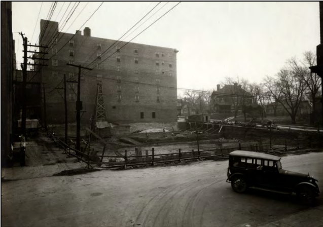
Figure 7: Excavation for the Warden Shops and Apartment Building, November 21, 1922. Photo taken from alley between 10 th St. South and 9 th St. South; view facing southeast. The Wahkonsa Annex can be seen in the background of the construction site.
