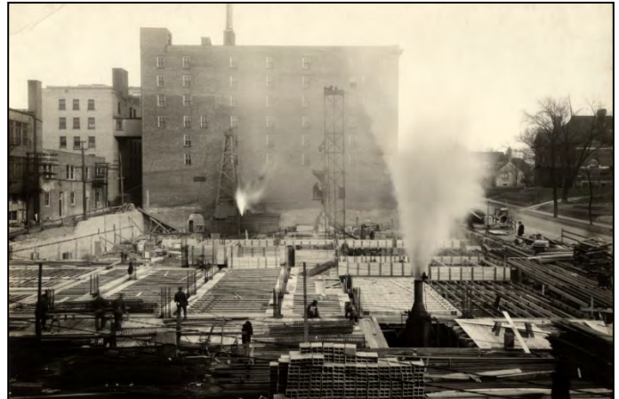
Figure 8: Construction of basement and first floor of the Warden Shops and Apartment Building, December 29, 1922. Photo taken from 9 th St. South; view facing east.
