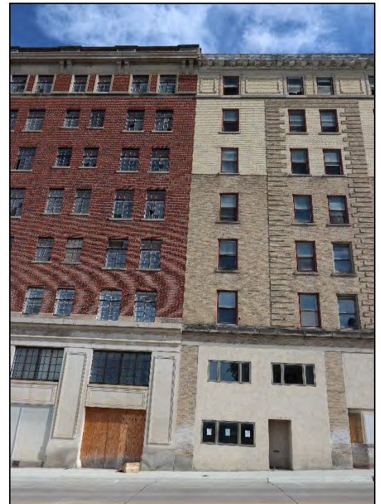
Figures 15 & 16: Exterior views of where the Warden Shops and Apartment Building abuts the Wahkonsa Annex. Notice cornice details are not consistent between the two buildings. Source: Strata Architecture, 2017
