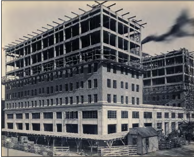
Figure 11: Construction photo of the Warden Shops and Apartment Building, November 1, 1923. Photo taken from the corner of 9 th St. South and 1 st Ave. South; view facing northeast. Source: Webster County Historical Society
