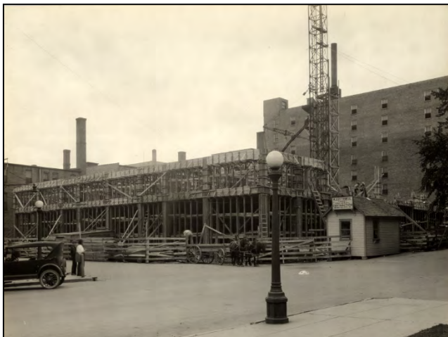
Figure 9: Construction of first and second floor of the Warden Shops and Apartment Building, June 23, 1923. Photo taken from the corner of 9 th St. South and 1 st Ave. South; view facing northeast. The Zitterell Construction Company's sign can be seen on the small shed.
