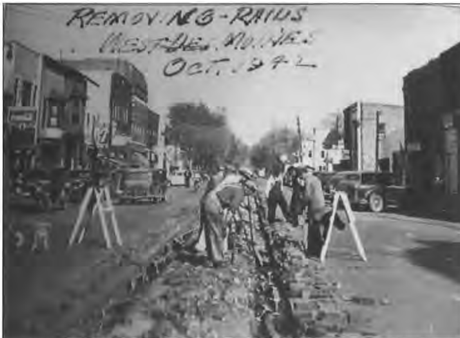
Figure 103: Interurban track removal, further south in 200s block looking north (Jordan House Library and Archives)
