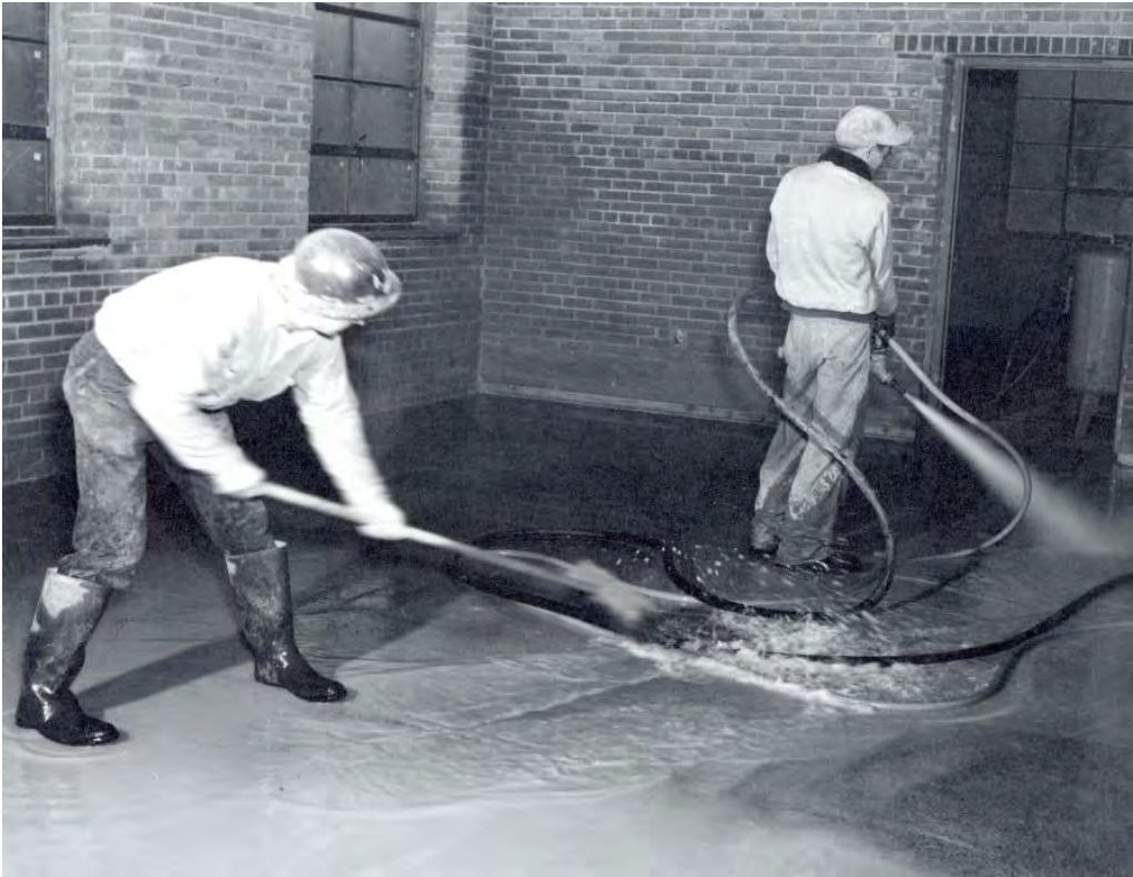
Clean-up crew cleaning structural concrete after sandblasting in preparation for placing bonded concrete floor topping in the Ephrata Office Building. Reclamation Photograph No. 4-4681, January 3, 1951.
