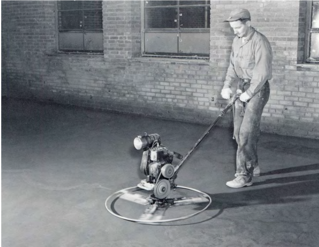
Concrete finisher operating power troweling machine on bonded concrete floor topping in the Ephrata Office Building. Reclamation Photograph No. 4-4679, January 3, 1951.
