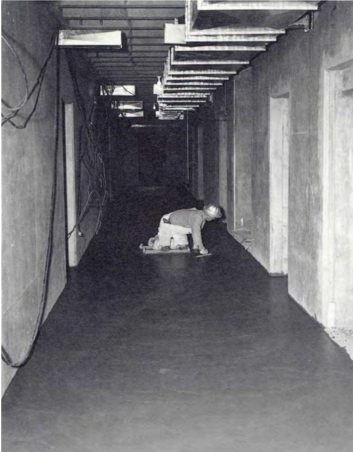
Concrete finisher finishing the floor in the basement corridor. Note ductwork at top of picture. Reclamation Photograph No. 4-4489, October 10, 1950.
