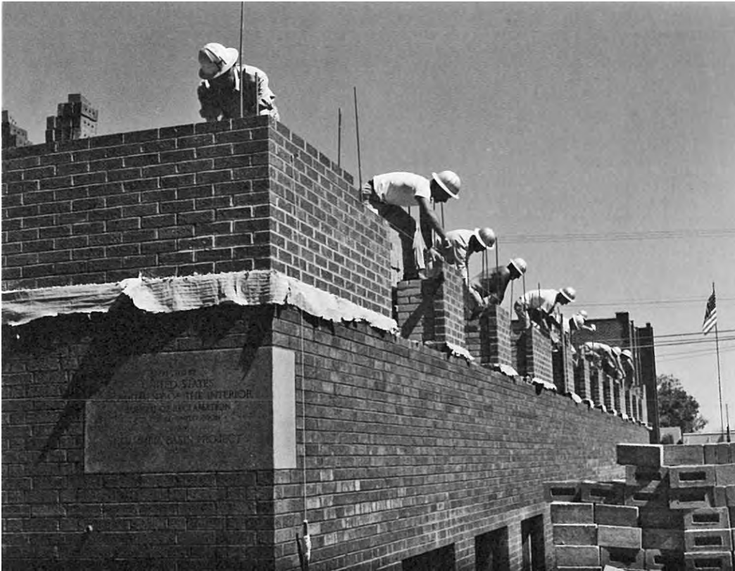
Brick masons working on the first floor of the Ephrata Office Building. Approximately 950,000 bricks are required. Reclamation Photograph No. 4-4183, August 3, 1950.
