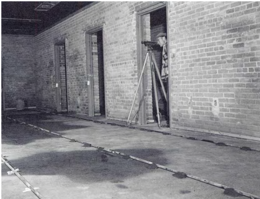
Instrument man leveling screeds in preparation for placing bonded concrete floor topping in the Ephrata Office Building. Reclamation Photograph No. 4-4680, January 3, 1951.
