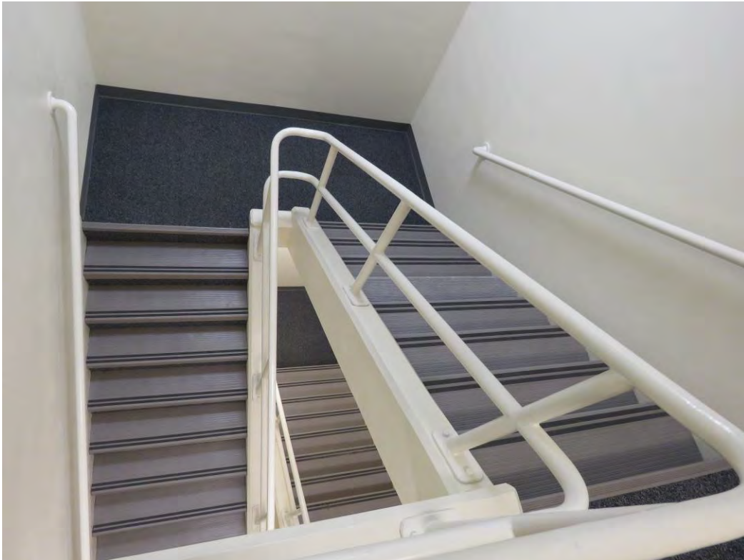
Photo No. 19 – Columbia Basin Project Irrigation Division Headquarters Office – South stairwell looking down from Third Floor.
