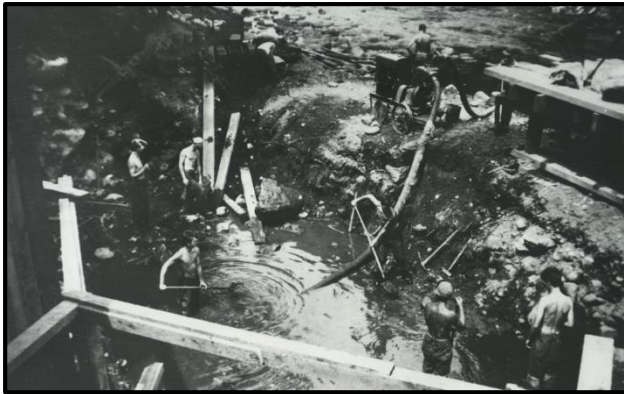
Figure 39. CCC men from Camp Speculator building the bridge at Speculator Campground, late 1930s. Adirondack Museum.
