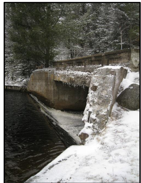
Figure 44. Dam on Rock Creek, Lake Durant Campground, Blue Mountain Lake, NY, 2016.
